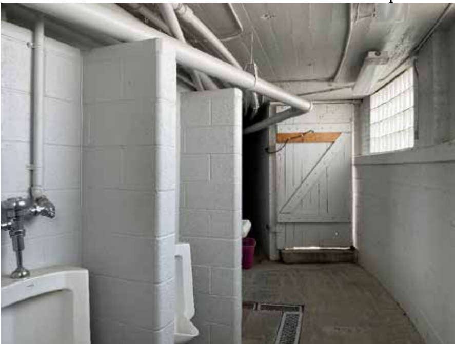
Photo 16: View of men's locker room and wooden door to pool deck stairs. Camera facing west.
