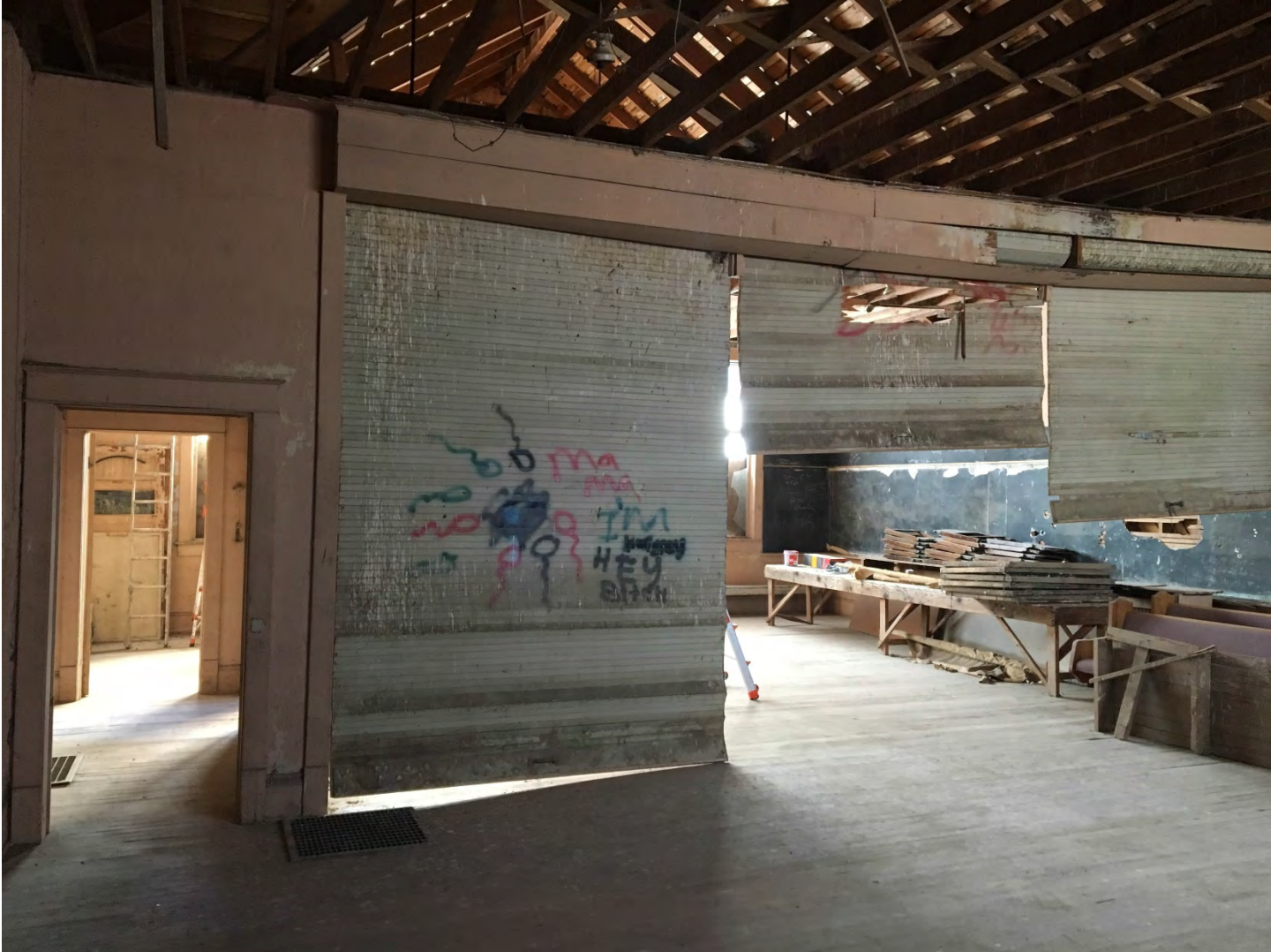
Photo 15 of 18: ID_TwinFallsCounty_RogersonSchool_0015 Interior, partition between east and west classroom space, looking east
