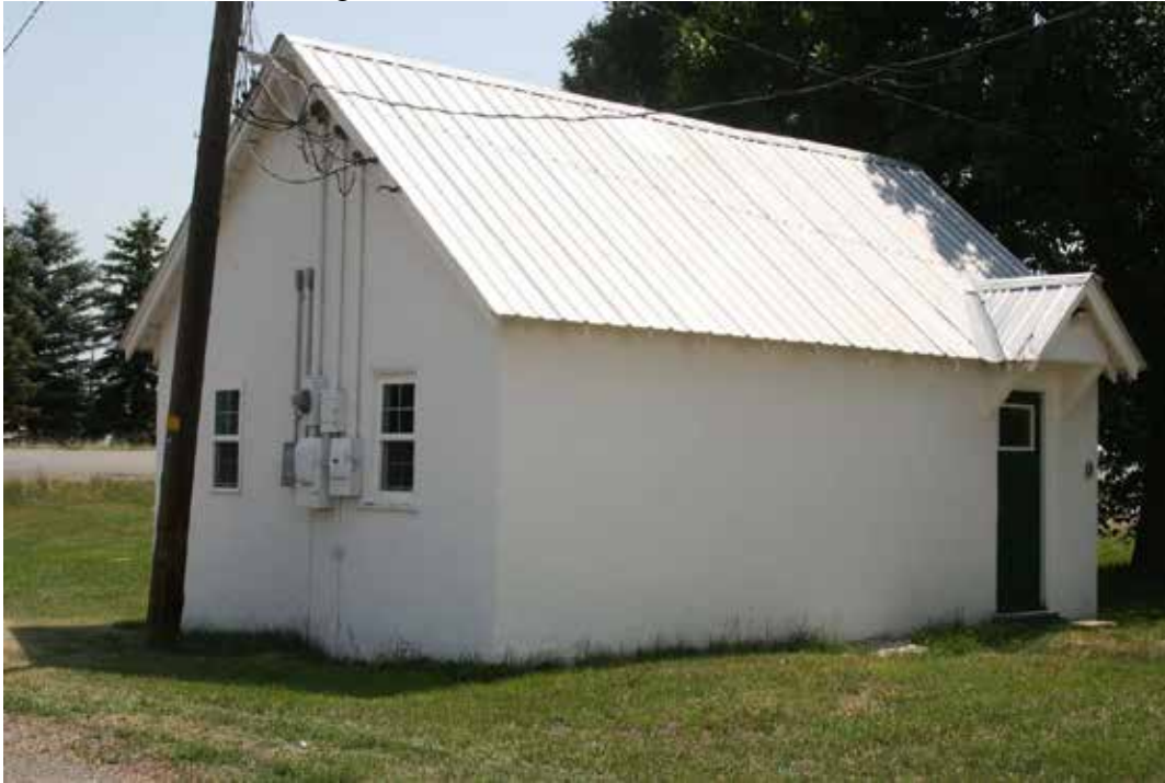
Photo 33: Stucco Cottage 1 (resource 13), view of north and west elevations. Camera facing southeast.
