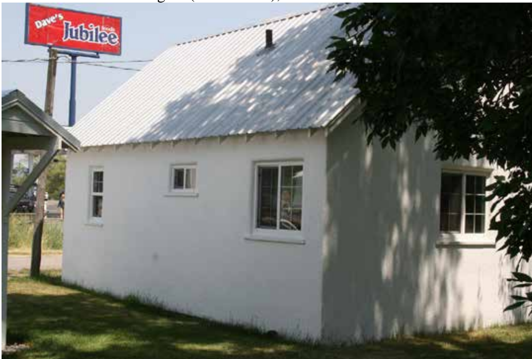
Photo 36: Stucco Cottage 2 (resource 14), view of west and south elevations. Camera facing northeast.
