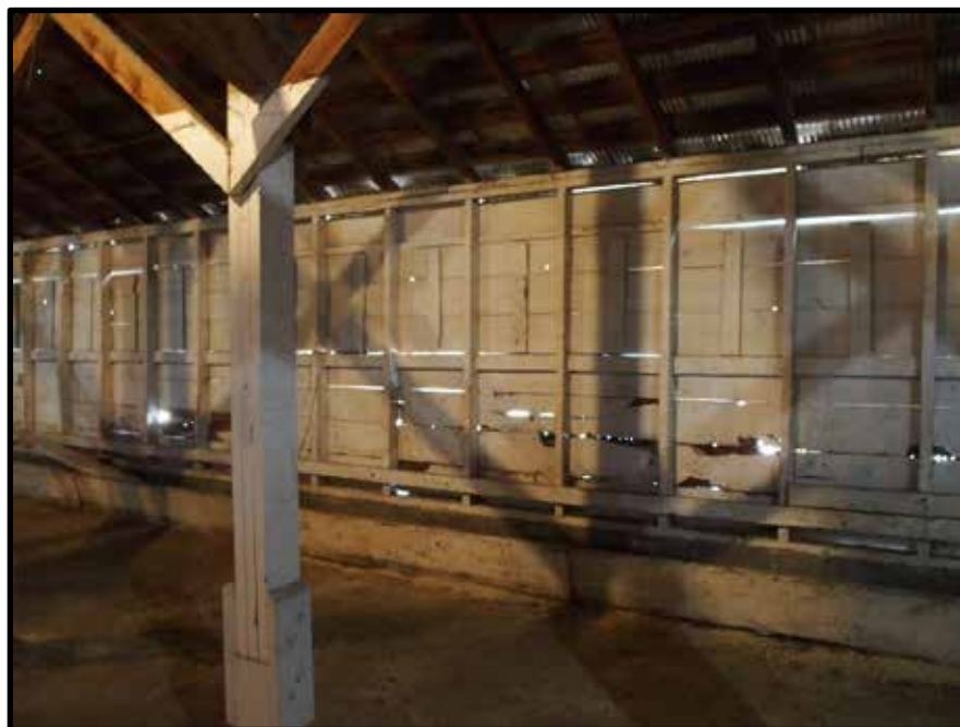
Photo 34 of 63: Interior of Resource 16 showing windows and feeding trough on north wall. Camera facing northwest.
