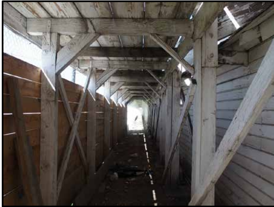
Photo 35 of 63: View of Resource 16 showing walkway below bleachers and south elevation of Dairy Barn. Camera facing west.
