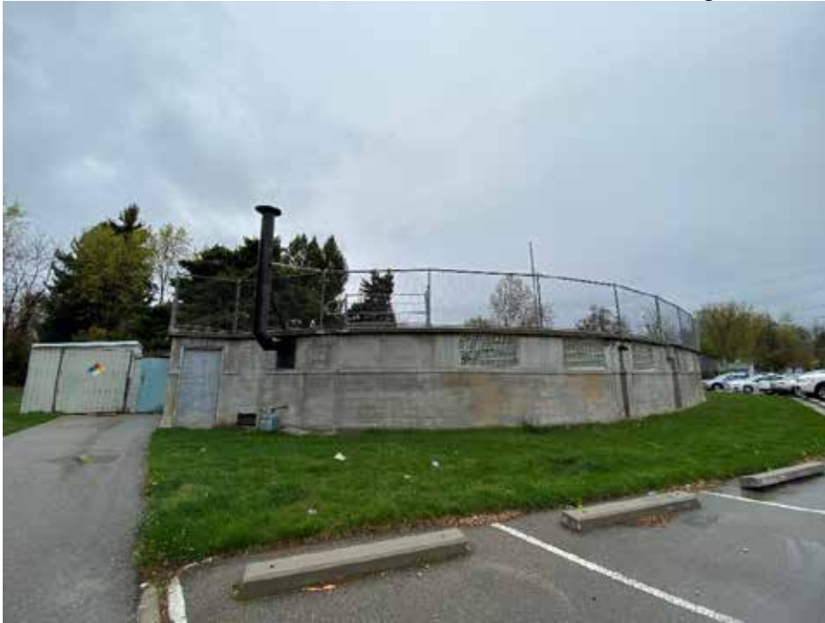
Photo 10: View of side (south) elevation with attached storage sheds. Camera facing north.
