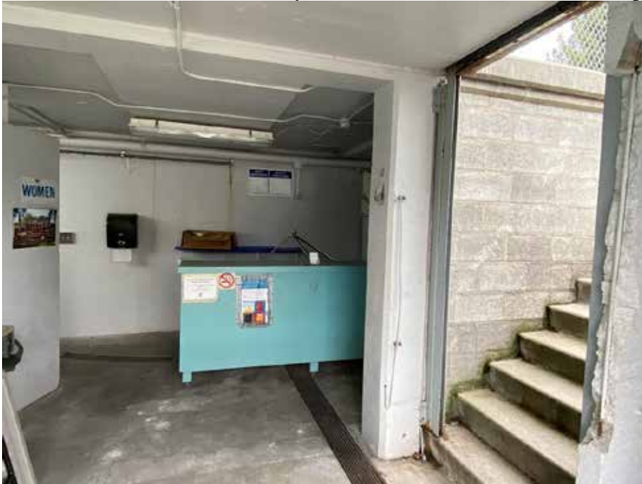
Photo 14: View of check-in lobby and entrance vestibule with stairs to pool deck. Camera facing west.
