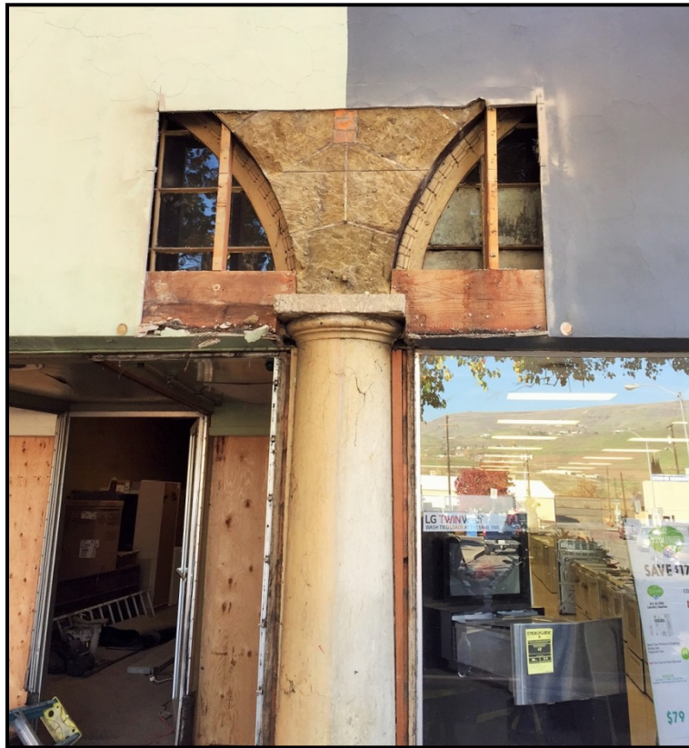
Figure 10. Original columns and arched transom lights discovered in November 2016 beneath a stucco and tile update of the Largent's (Resource Number 11) façade (photograph courtesy of Jacqui Gilbert, City of Lewiston).
