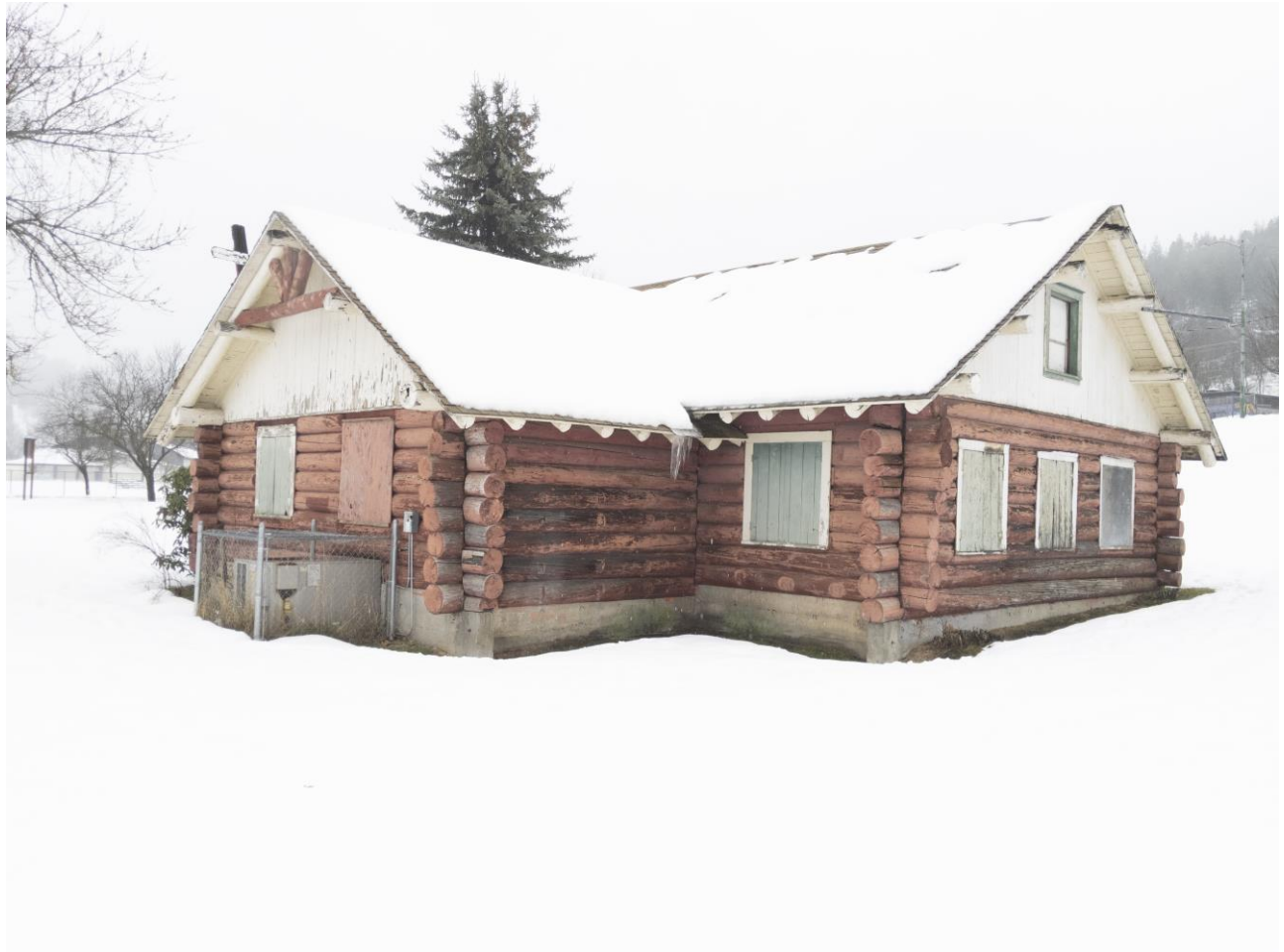
Photo #4: View of north (left) and west (right) elevations. Camera facing southeast.
