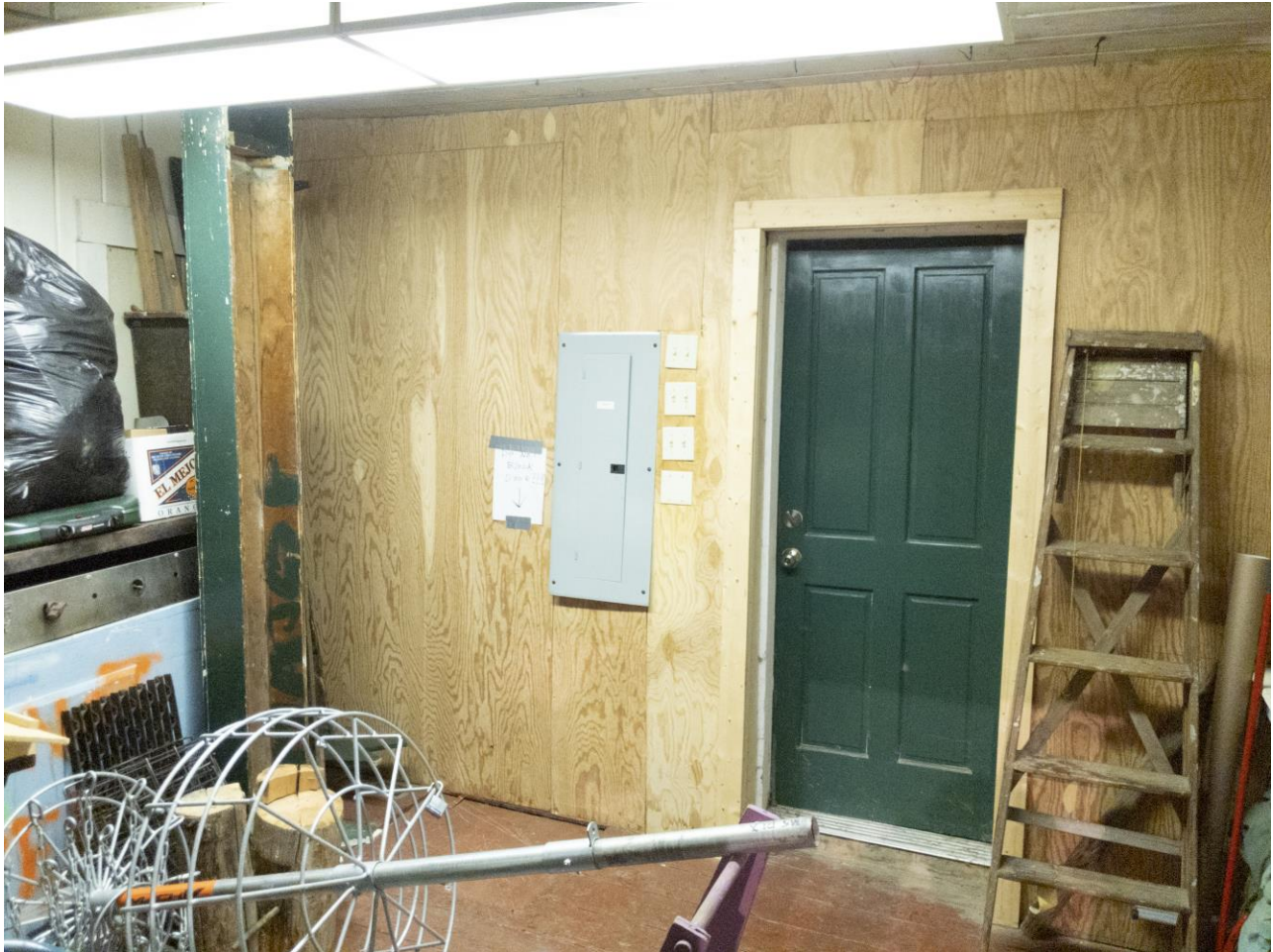
Photo #14: View of plywood covered wall and exterior door in storage room. Camera facing south-southeast.
