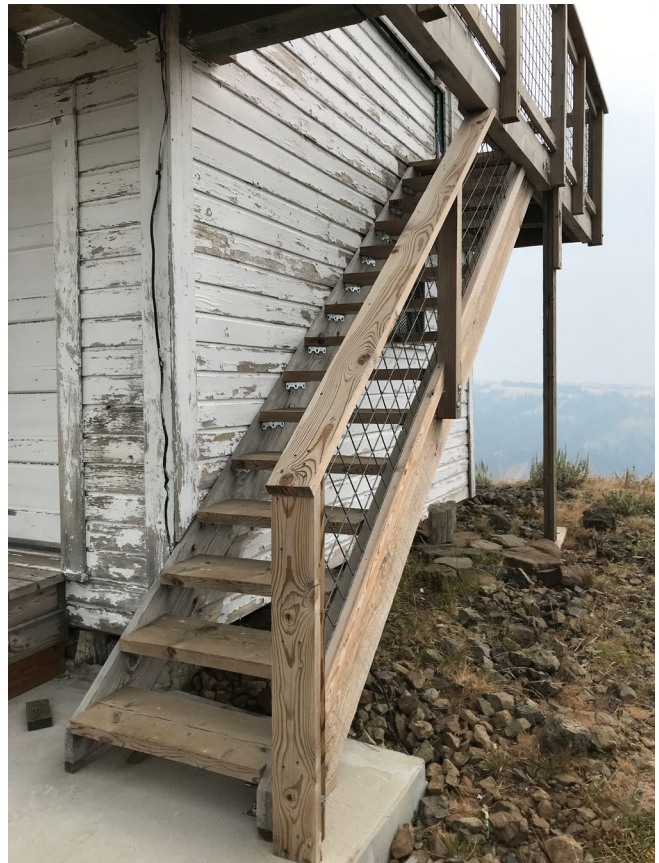
Photo #22. Stairs (restored 2019) to catwalk and lookout cab. Southwest corner. Facing northeast.
