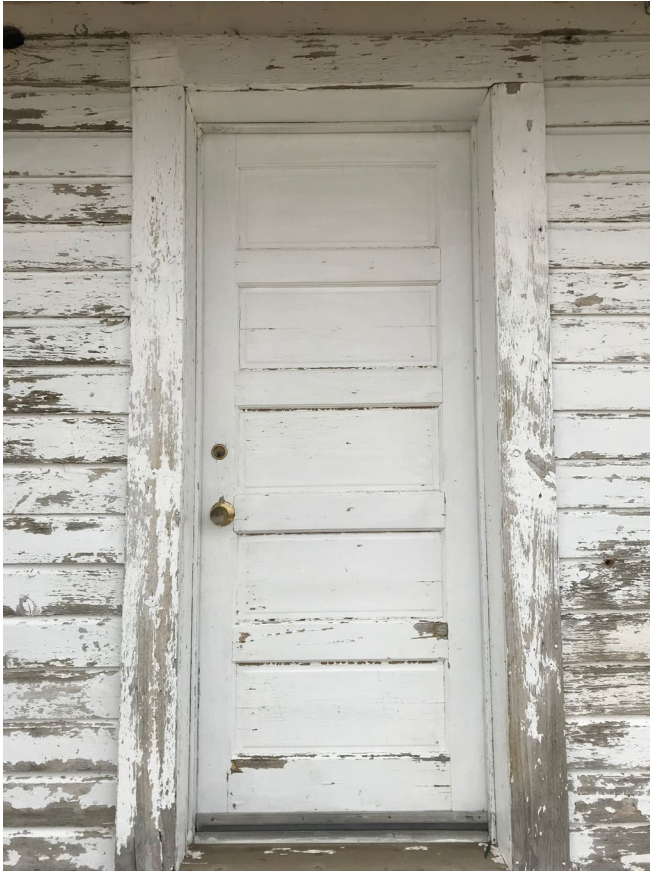
Photo #21. Historic Lookout. Door to one room substructure (storage) Facing west. East elevation.
