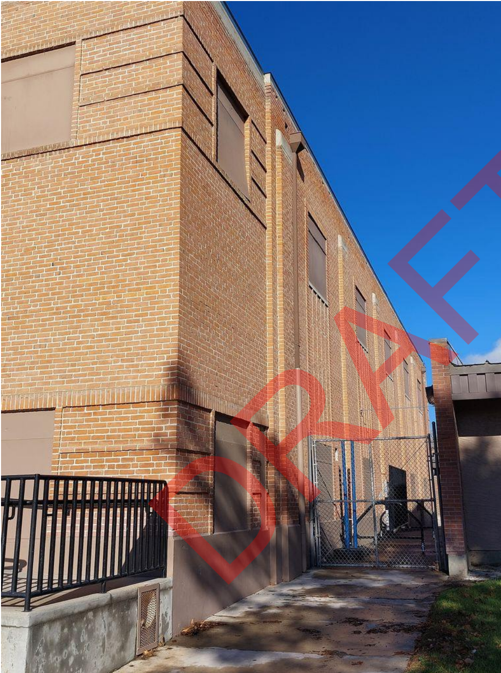
Photo 4 of 26. ID_Washington_WeiserHighSchoolGymnasium-Auditorium_0004 View of east side elevation with adjacent middle school building at left, camera facing north
