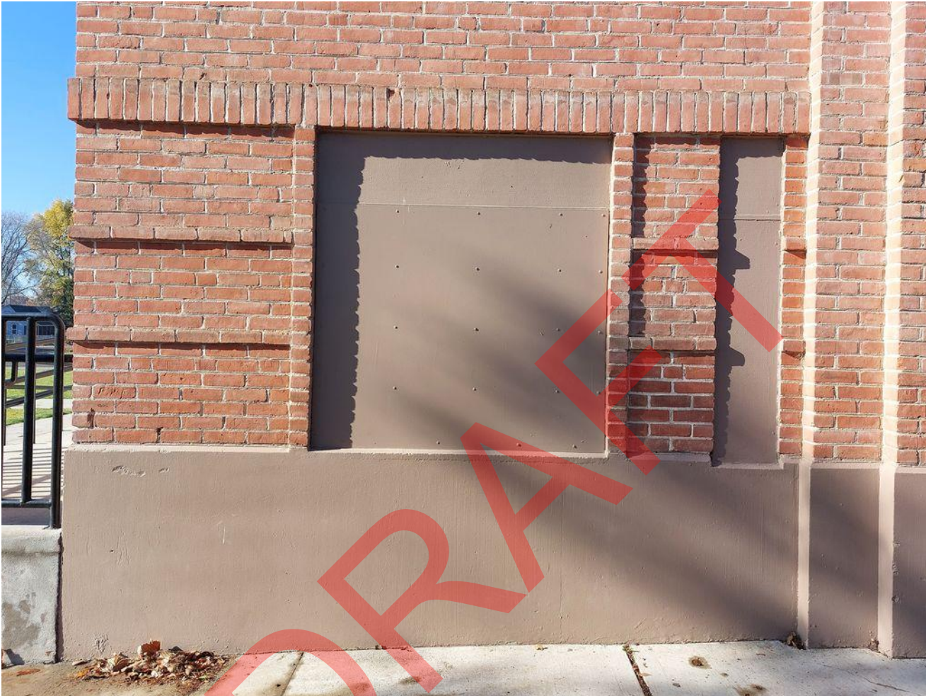
Photo 5 of 26. ID_Washington_WeiserHighSchoolGymnasium-Auditorium_0005 View of covered window at southeast corner, camera facing west
