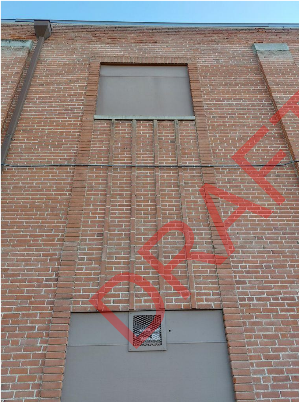
Photo 7 of 26. ID_Washington_WeiserHighSchoolGymnasium-Auditorium_0007 View of brick detail on west elevation, camera facing east
