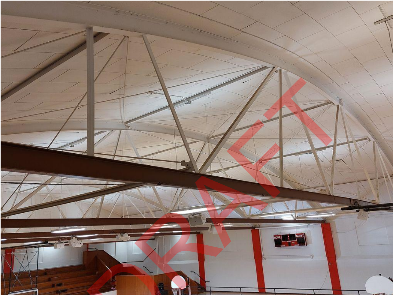
Photo 18 of 26. ID_Washington_WeiserHighSchoolGymnasium-Auditorium_0018 View of steel arch trusses supporting the roof, camera facing southwest
