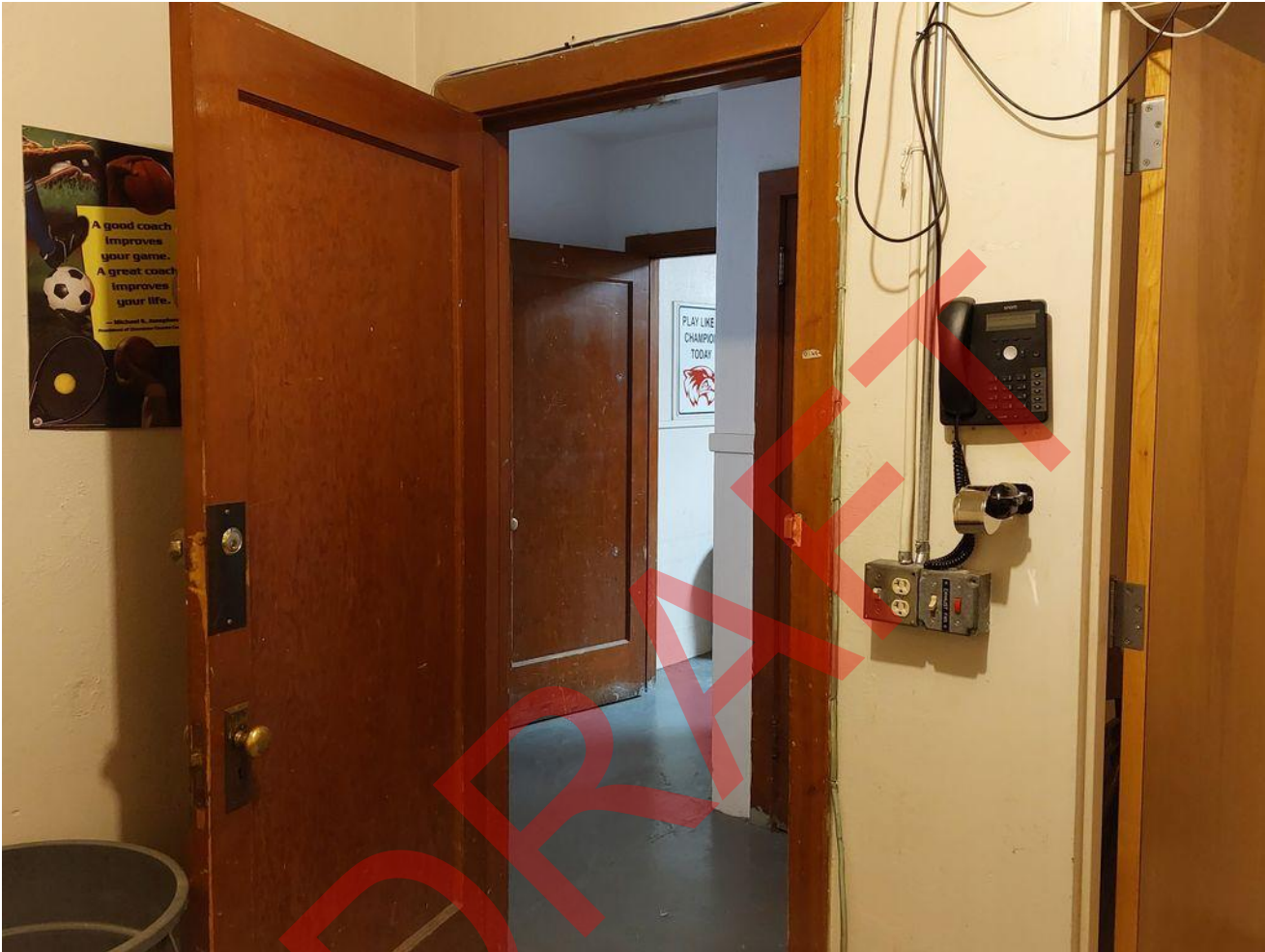
Photo 23 of 26. ID_Washington_WeiserHighSchoolGymnasium-Auditorium_0023 View from coach's office toward boys' locker room, camera facing northwest
