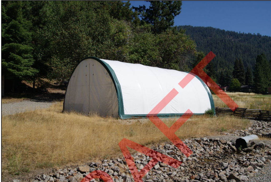
Photo 72. Arched canvas storage structure (resource 6) north of Memorial Hall, south and west elevations, view northeast. 2025.
