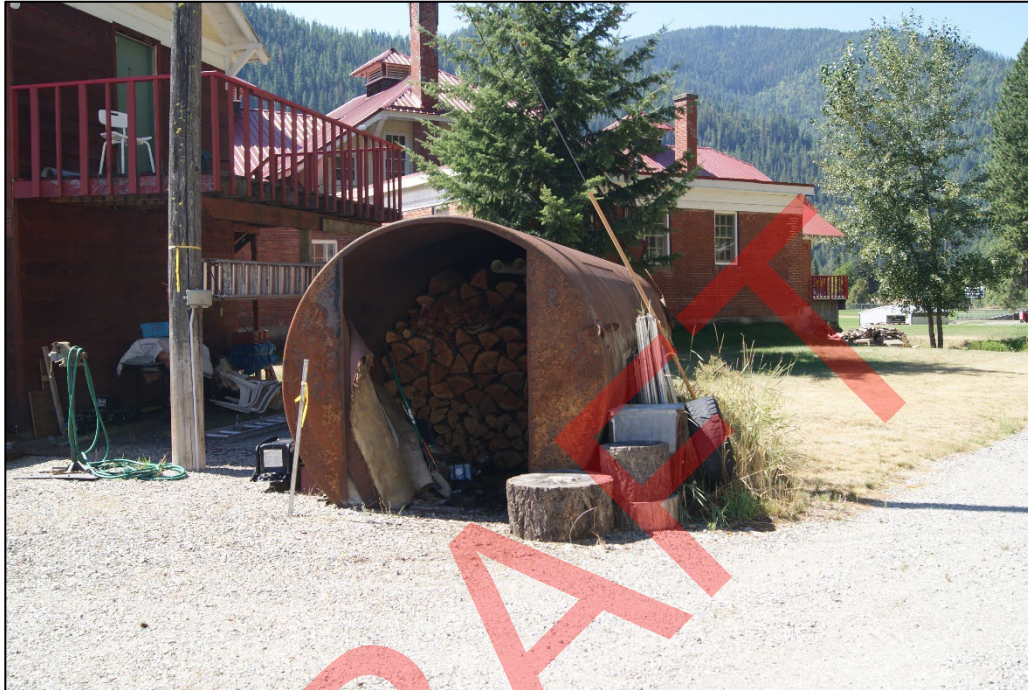
Photo 70. Memorial Hall oil tank (resource 5), northeast elevation, view south. 2025.
