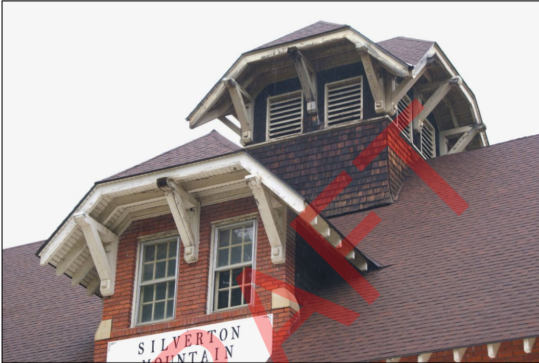
Photo 13. Infirmary (resource 1), central gable and roof cupola detail, south elevation, view northwest. 2024.
