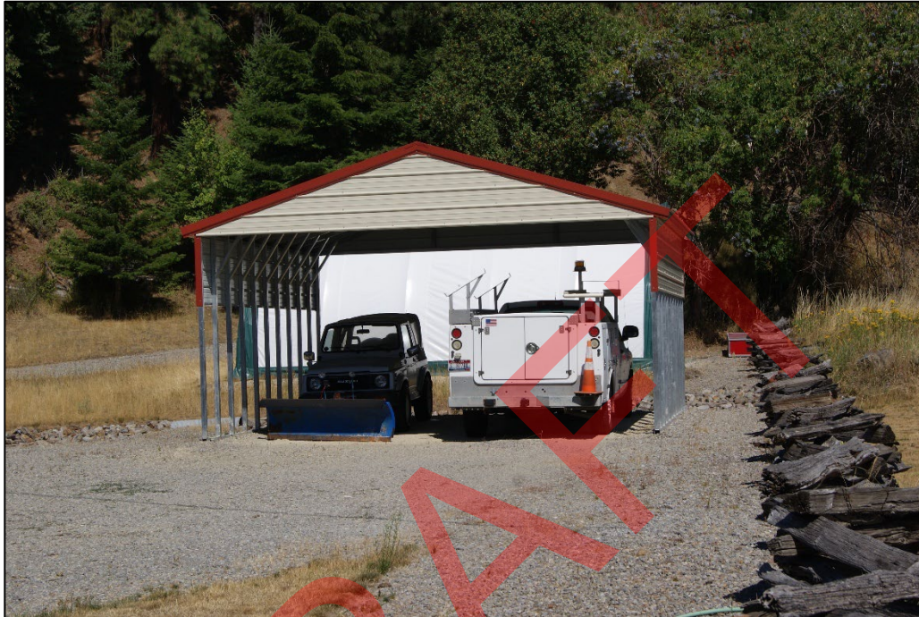
Photo 73. Steel vehicle shelter (resource 7) northeast of Memorial Hall, south elevation, view north. 2025.
