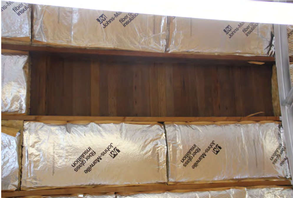
Photograph 34. Interior, Second Floor, detail view of cedar ceiling material above the added insulation in Legion Hall. Camera facing north.
