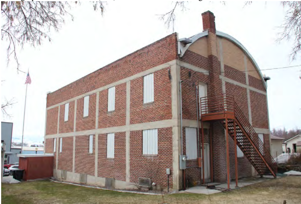
Photograph 8. Exterior, oblique view of east (rear) elevation and south elevation. Camera facing northwest.
