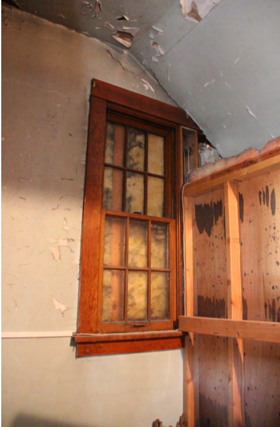
Photograph 35. Interior, first floor, blocked in window under the stairway. Camera facing south.
