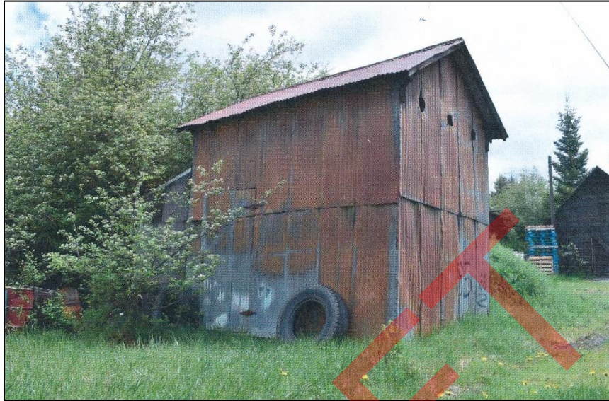
Outbuilding in rear yard, east side and front (north) facades, looking southwest
