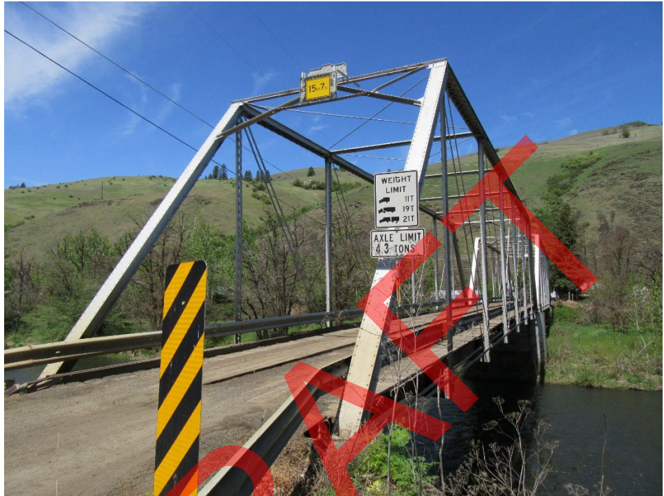
Photo 3. View of the Sperry Bridge from the south bank of Potlatch River looking northwest.
