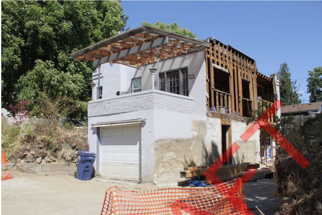
9. House at 901 E. Montana Ave. undergoing heavy alteration in summer 2023. Camera facing northeast.
