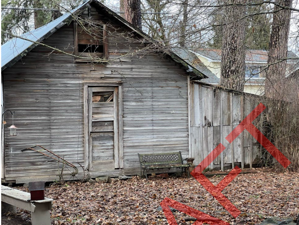
99. The outbuilding at 819 E. Pennsylvania Ave. was known to be an icehouse. Camera facing south.
