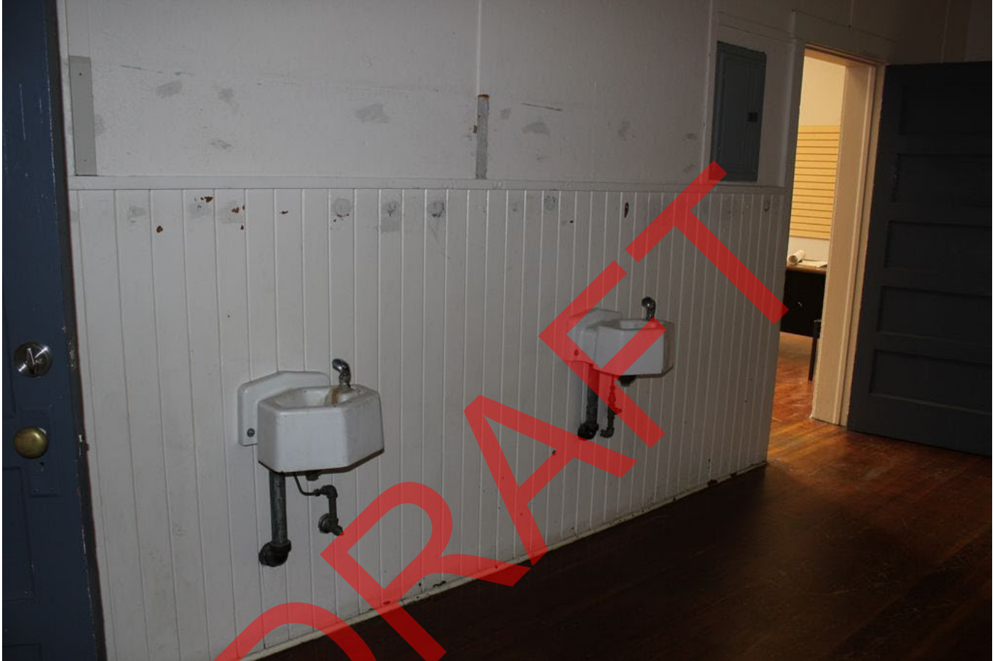
Photo 14 of 21. ID_IdahoCounty_RigginsHighSchool_0014 Water fountains along center corridor wall on the main floor (now non-functioning).
