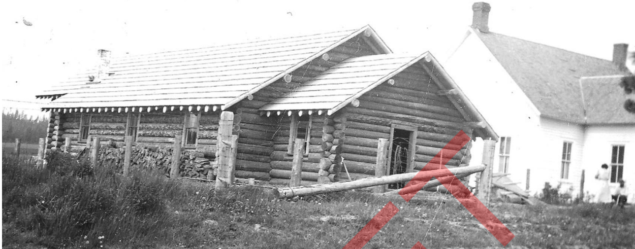
Evergreen Grange under construction, with North Teakean School to the right (east). Ca. 1938.
