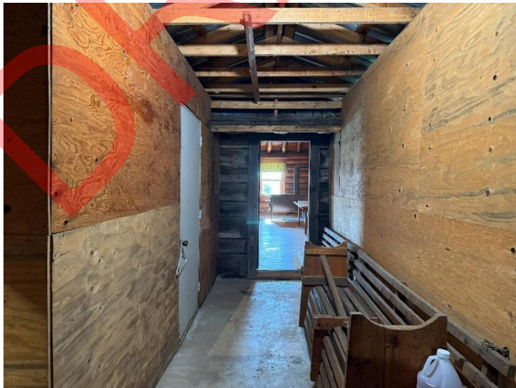
Photo 60: Hallway connecting Evergreen Grange Hall to the north façade of the Fire Hall. Restrooms located off hallway, facing west. (DE photo)
