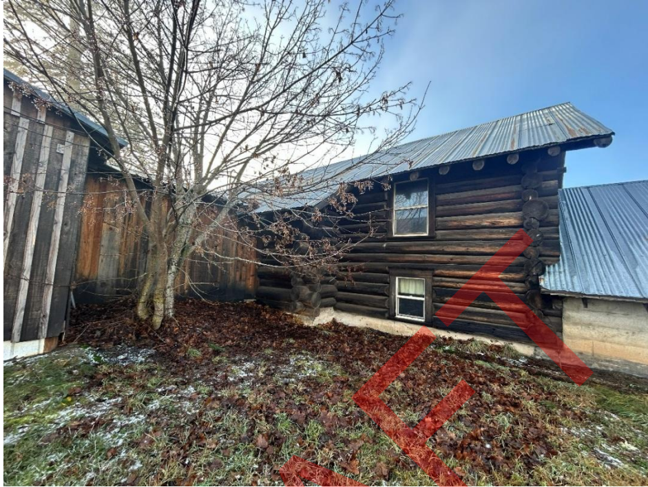
Photo 11: Detail photo of rear and side elevation showing connection to fire hall.
