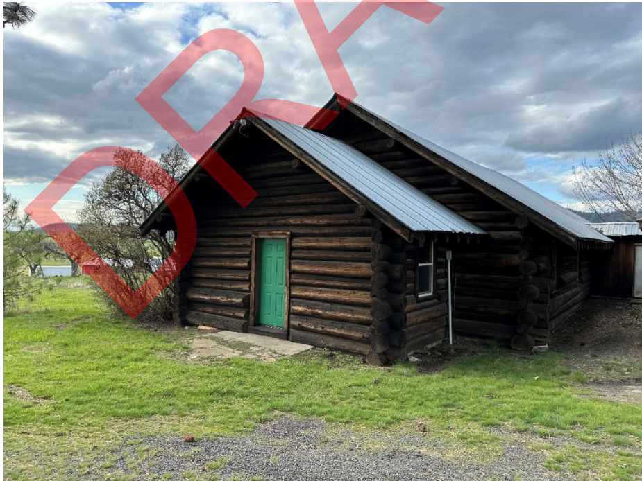
Photo 4: Detail photo of entrance area, showing where light used to be. (DE photo)
