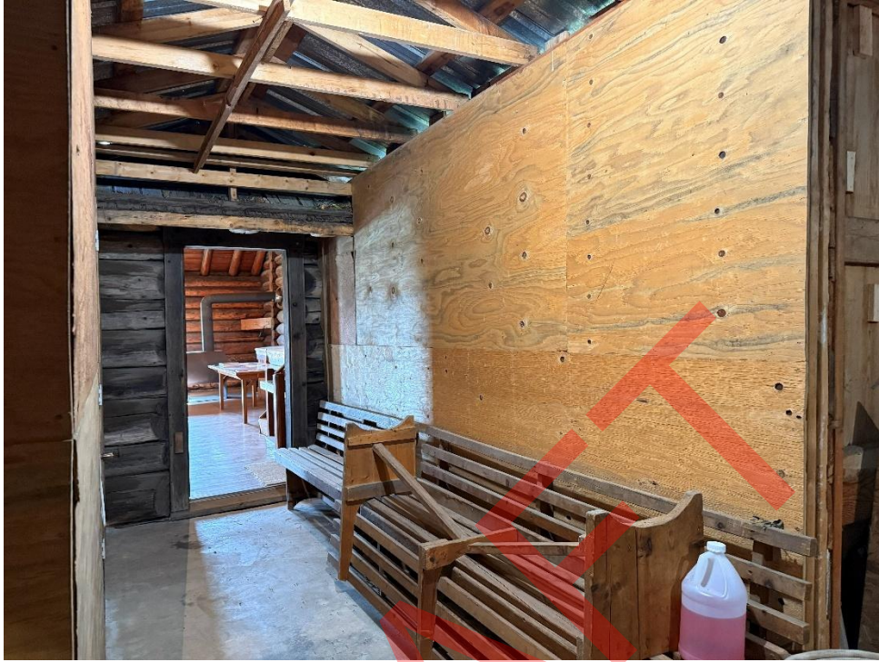
Photo 61: Hallway connecting Evergreen Grange Hall to the north façade of the Fire Hall, facing west by west northwest. (DE photo)
