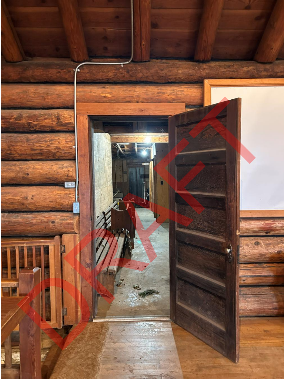
Photo 45: Door on east wall of Evergreen Grange Hall leading to restrooms in vestibule behind the Fire Hall.
