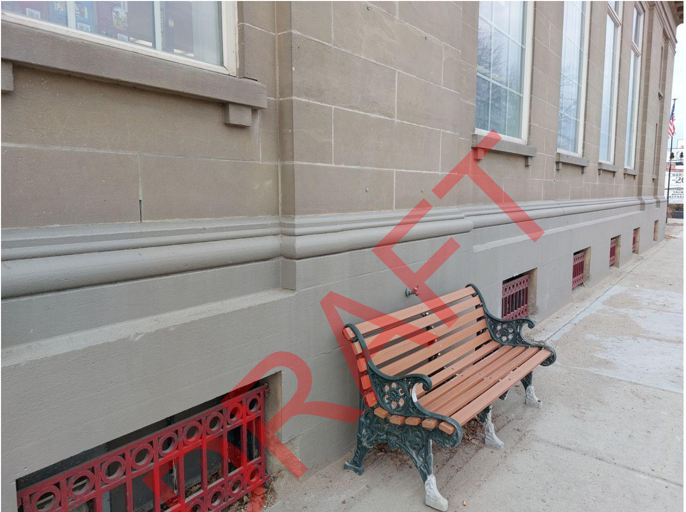
Photo 7 of 24. ID_Canyon_ParmaStateBank_0007 View of foundation level on north elevation, camera facing southwest
