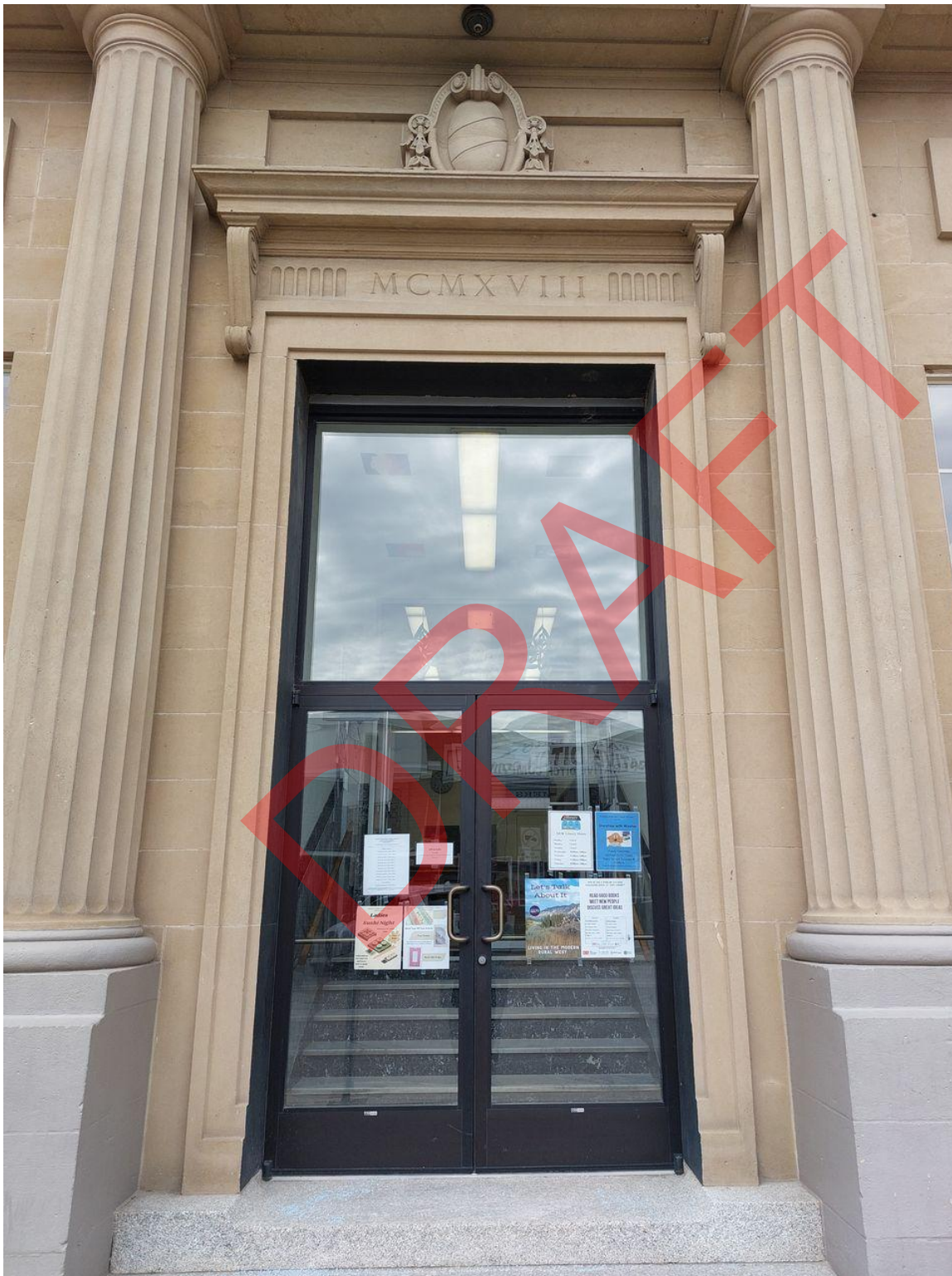
Photo 9 of 24. ID_Canyon_ParmaStateBank_0009 View of primary entrance on east elevation, camera facing west
