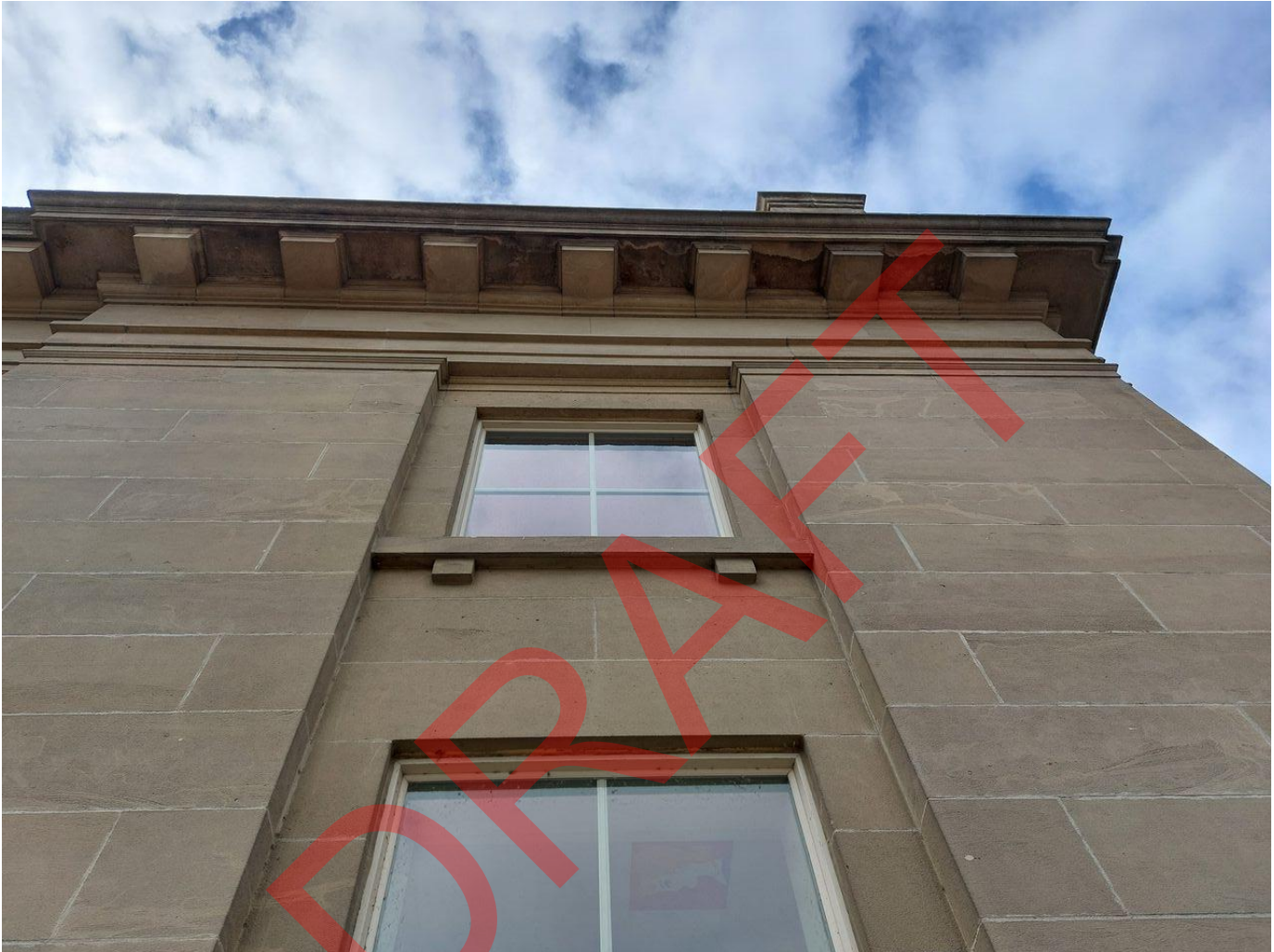
Photo 5 of 24. ID_Canyon_ParmaStateBank_0005 View of roof and windows on north elevation, camera facing south
