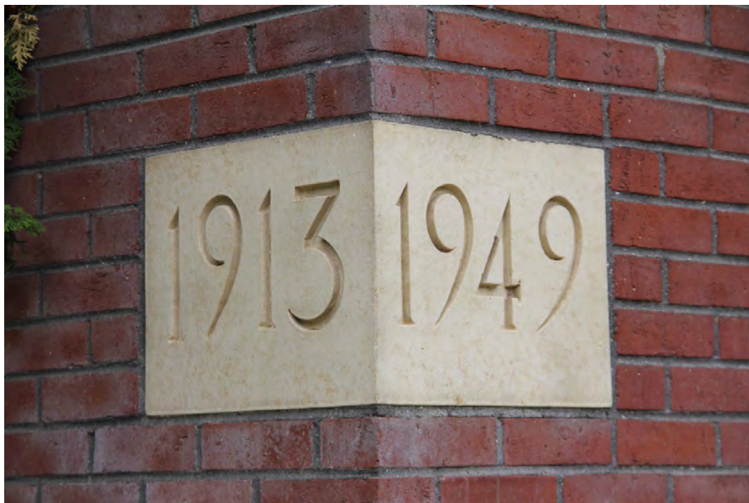
Photograph 12. Exterior, cornerstone detail on north (main) and east facades. The 1949 date marked the beginning of construction of the building and 1913 is the founding date of the congregation. Camera facing southwest.
