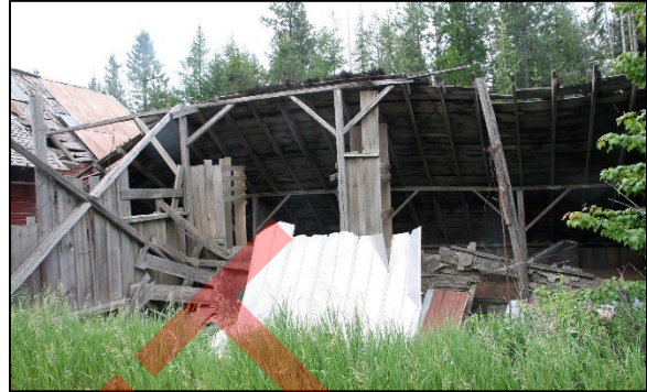
Figure 37. A partially collapsed barn at 10148 West Thompson Road.
