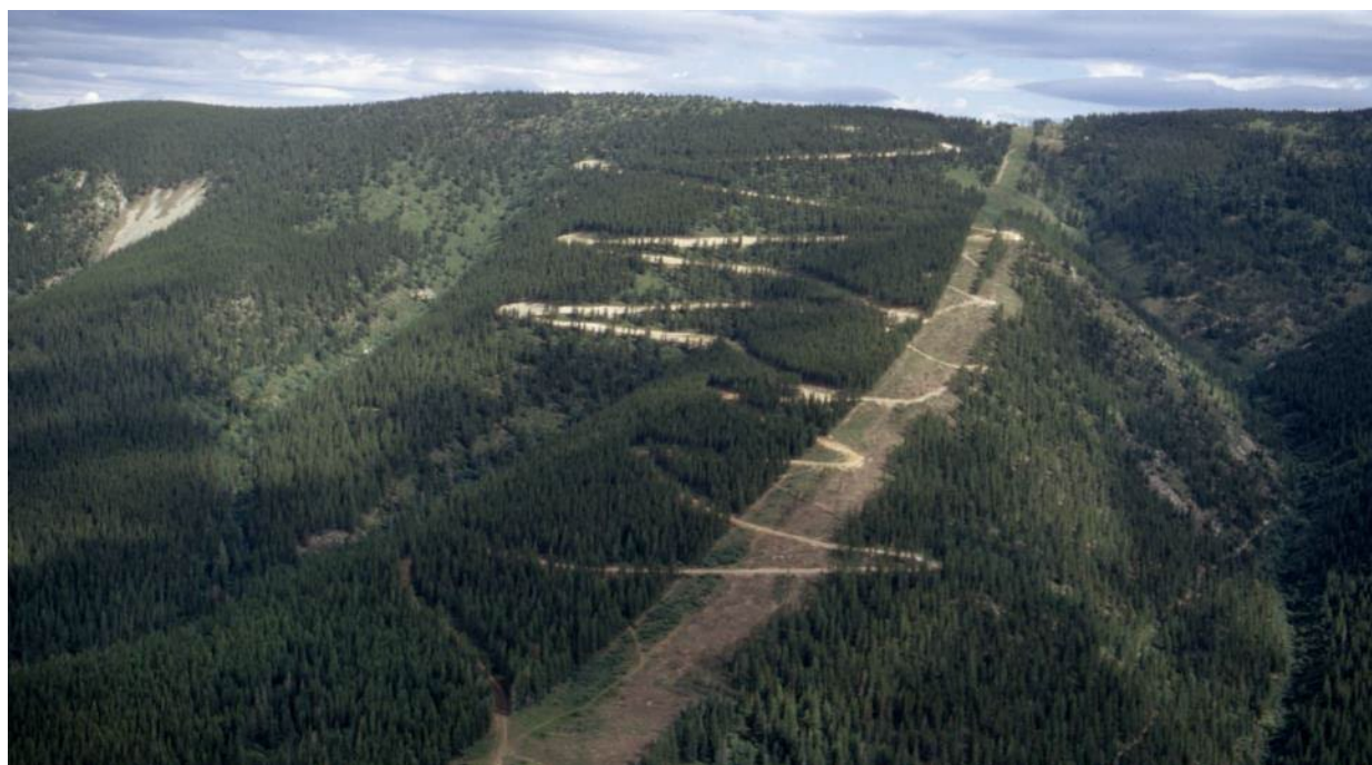
Figure 61. Clearing the right-of-way and access roads for the construction of the Dworshak-Hot Springs Line, which was energized in 1973, date unknown. 343
