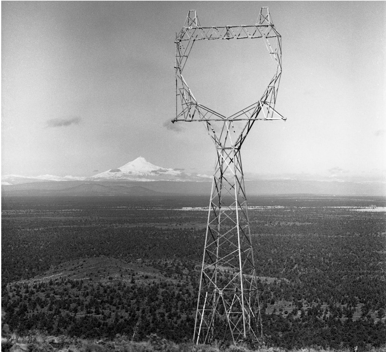
Figure 46. Construction of a Delta Configuration tower along the Pacific Direct Current Intertie near Bend, Oregon, October 1966. 292
