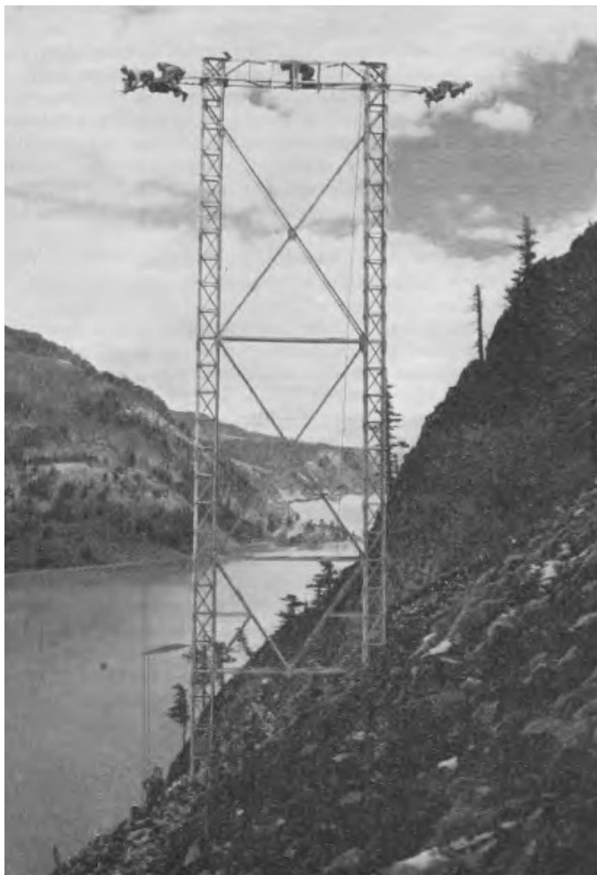
Figure 6. Line workers completing a high-tension transmission line in the Columbia River Gorge circa 1941. 29
