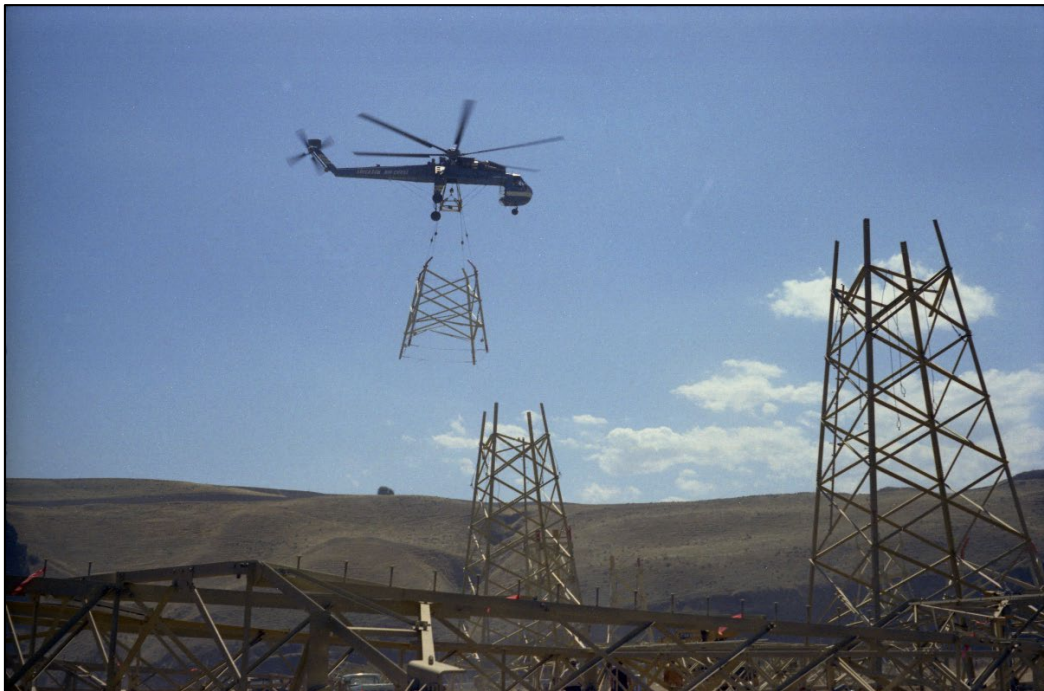
Figure 37. A sky crane is used to avoid scarring the hillside with access roads during installation of towers for the Lower Granite–Hatwai 500-kV Line near Lewiston, Idaho (1972). 258
