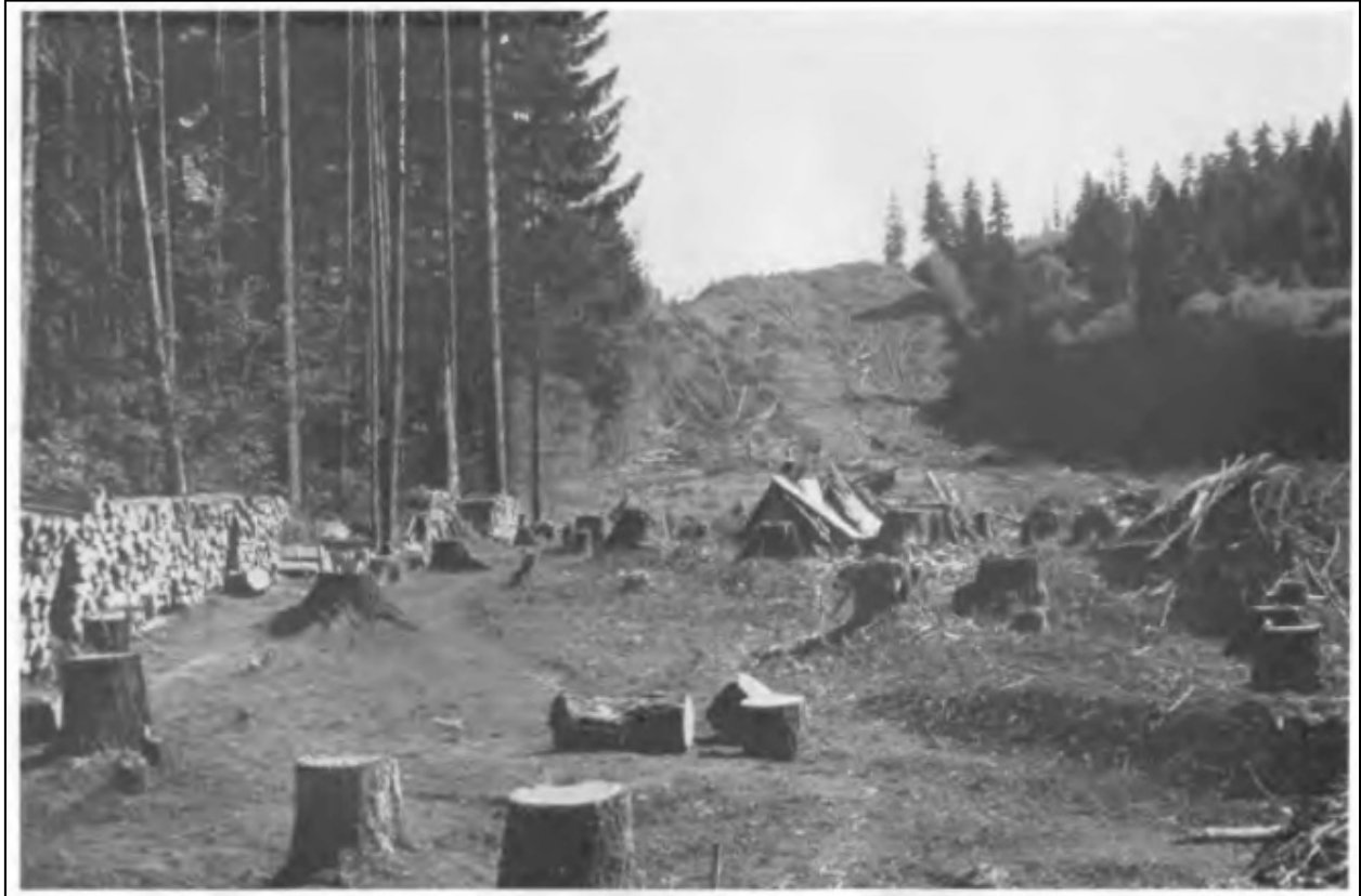
Figure 12. WPA crew members cleared these trees for the Kelso-Raymond Line right-of-way, June 13, 1939. 114
