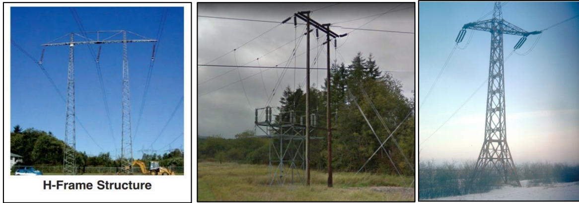
Figure 87. Unique Transmission Structure Types, including lattice steel H-frame structures (left), switch stands (middle) and single circuit direct current lattice steel structures (right), which are only used on direct current lines. 395
