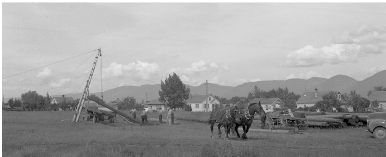
Figure 26. Horses help erect a tower in a rural residential area during the construction of the Hungry Horse-Kerr Dam 115-kV Line, ca. 1947. 181
