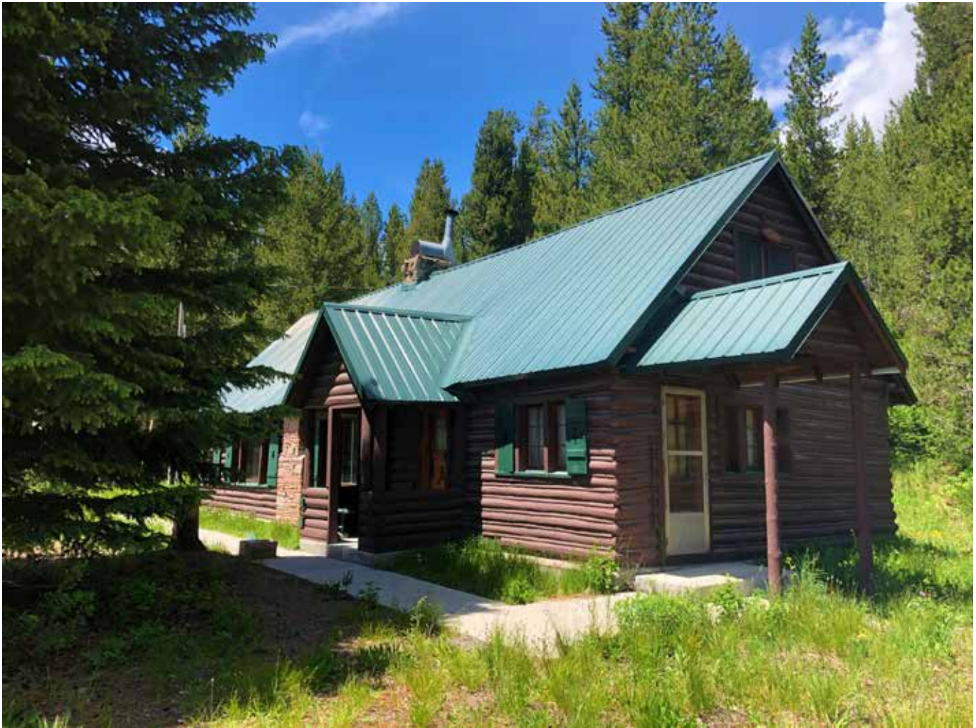
Photo 5. Cabin's south / front and east / side elevations looking northwest. East / side porch featured.
