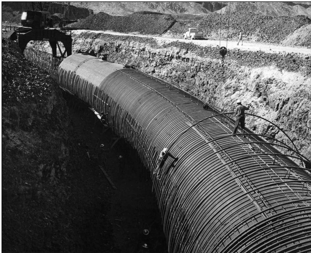
Figure 3.18 A portion of the Soap Lake Siphon steel piping being constructed, along with the reinforcing steel for the concrete portion. 177
