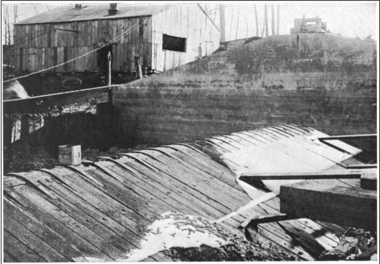
Figure 4.11 Southside abutment of the rock and timber covered diversion on the Lower Yellowstone River (1917), Lower Yellowstone Project (Montana, and North Dakota). 207
