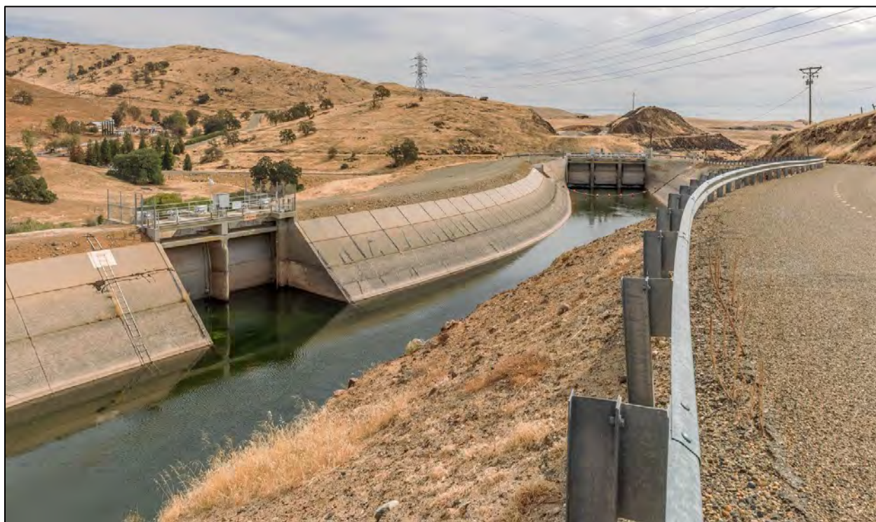
Figure 4.66 Concrete wasteway gate and wasteway on the Friant Kern Canal on the CVP (California). 257
