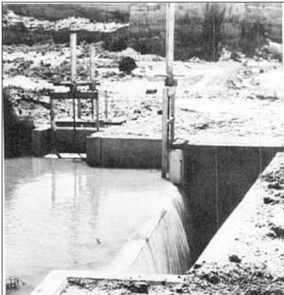
Figure 4.65 This photo shows an example of a concrete and iron gate wasteway gate and spillway. The gate is at the far end of the photograph. This particular style is called the side wastewater gate. 256
