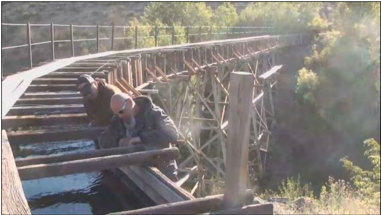
Figure 4.37 Wooden Flume # 13 in the Bitter Root Project (Montana) is an excellent example of a flume built in the 1930s and still operational today. 231
