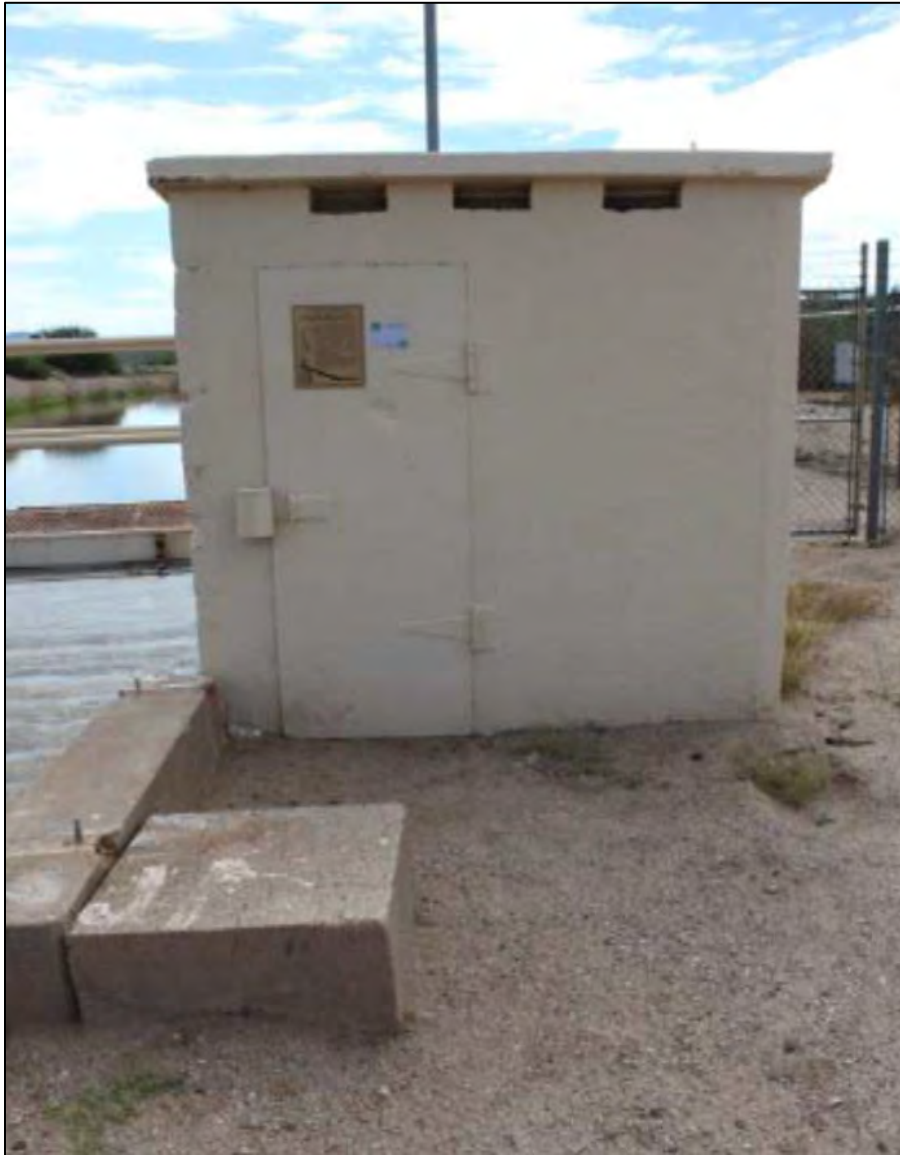
Figure 4.101 West façade of the stilling well in the Parshall flume of the Florence Casa Grande Canal in the San Carlos Irrigation Project (Arizona). 300
