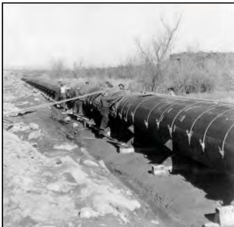
Figure 4.42 Wooden Stave Siphon being installed in 1941 on the Yakima Project (Washington State). 237
