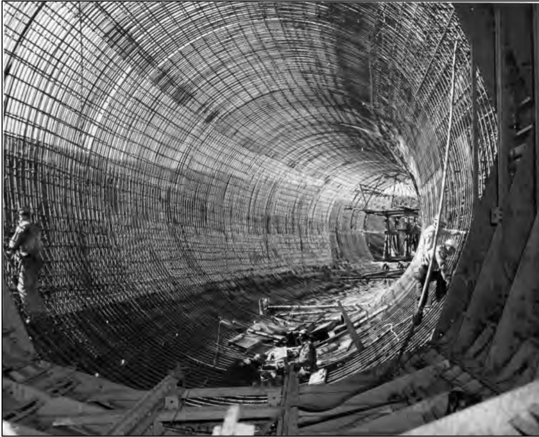
Figure 3.14 Large, lined canal of the Columbia River Irrigation project taken in the 1940s as it was being constructed. 168
