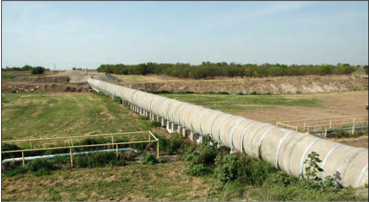
Figure 4.40 Concrete pipe flume in Hidalgo County Irrigation District on the Rio Grande Project (Texas). 234
