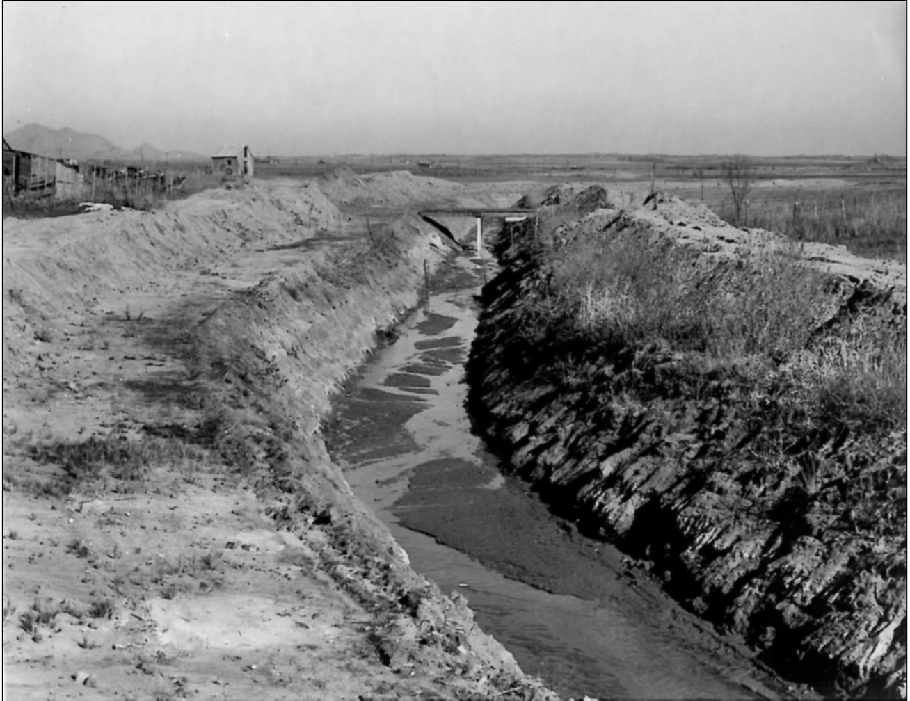
Figure 4.28 A typical example of an earthen drain in the W.C. Austin Project (Oklahoma). 225
