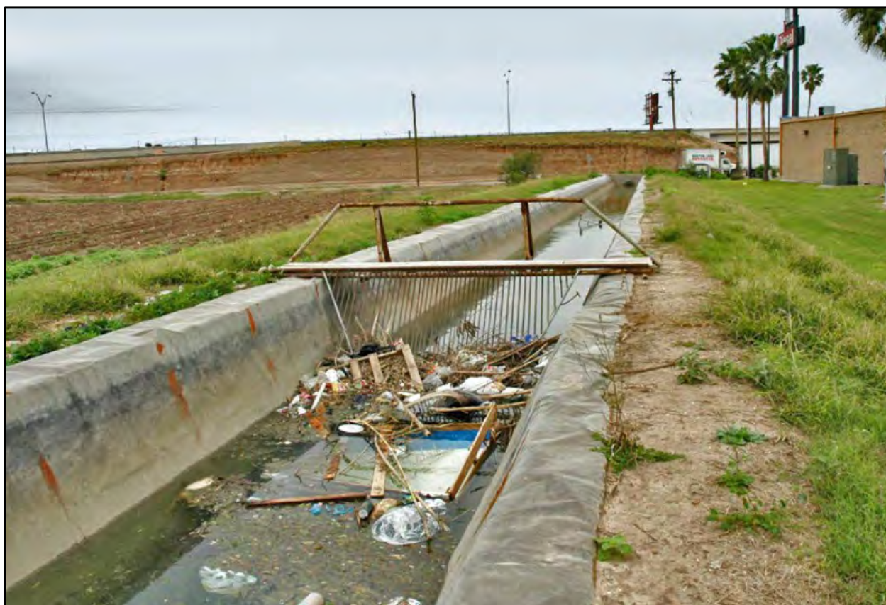
Figure 4.110 4.110 A trash rack in a lateral combined with a foot bridge in the Lower Rio Grande Project (Texas). 310
