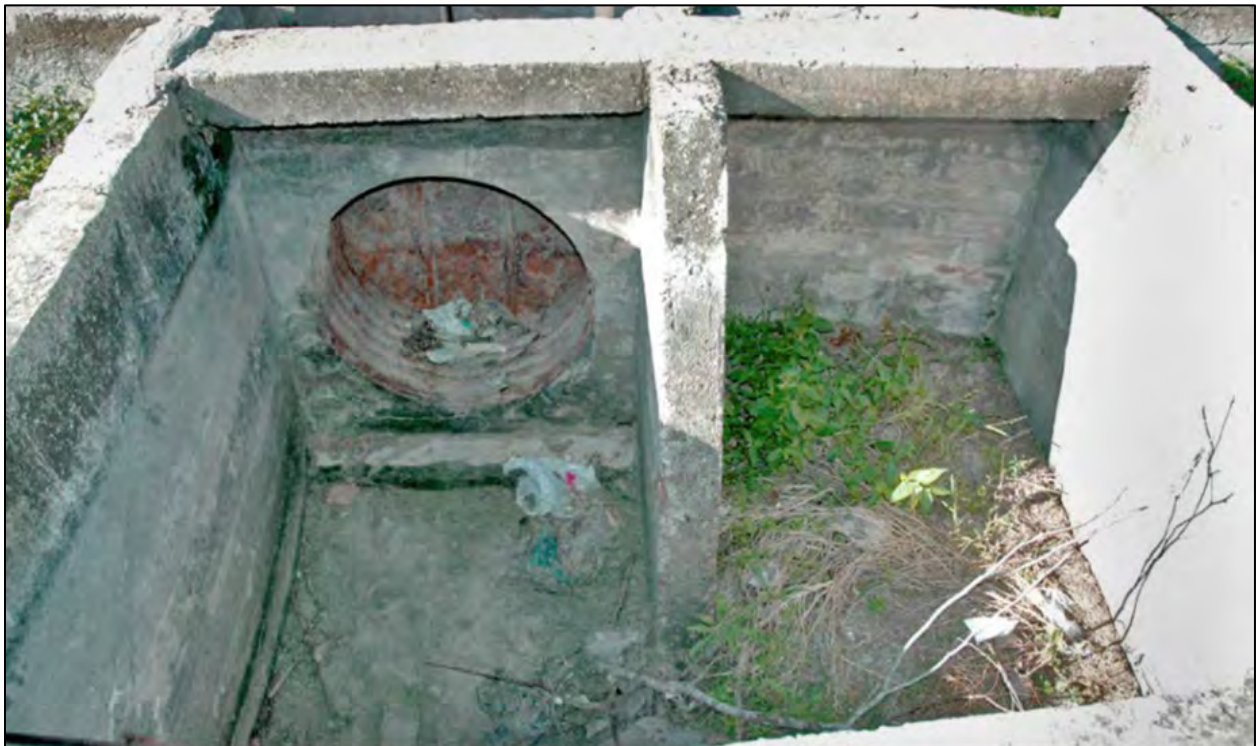
Figure 4.80 Interior of an underground concrete distribution box. 273
