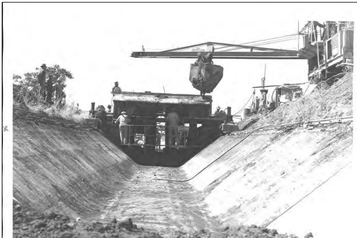
Figure 3.15 Contra Costa Canal. Lining operations on canal, 1948 (courtesy of Bureau of Reclamation).
