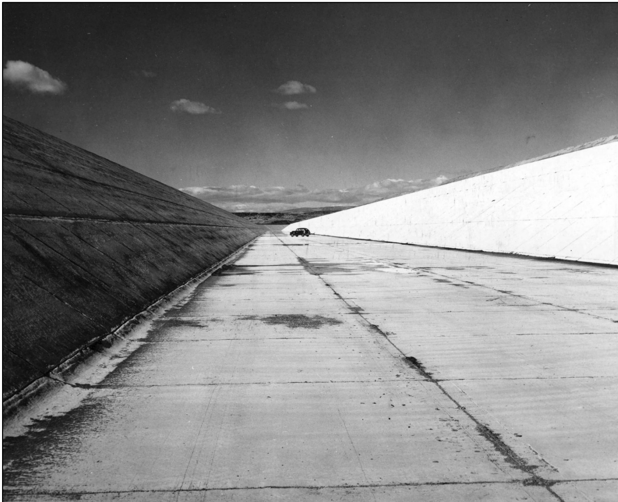
Figure 4.25 Main canals can vary widely in width and depth. The lined main canal in the Grant County Irrigation System portion of the Columbia River Basin Project (Washington State) is easily large enough for an automobile. 223
