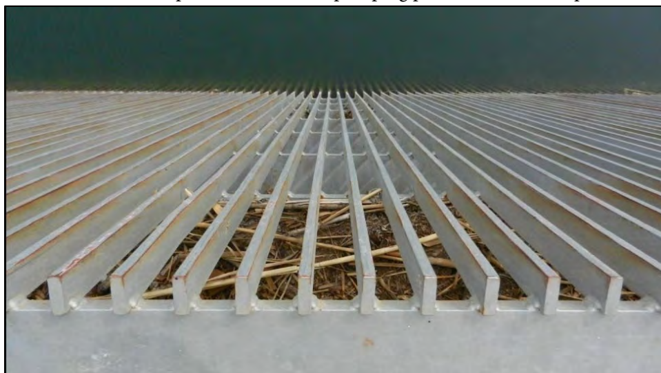
Figure 4.112 The style of trash rack used at the Senator Wash Pumping Plant, looking down on the rack from above, showing debris in the Colorado River Storage Project (Arizona). 312
