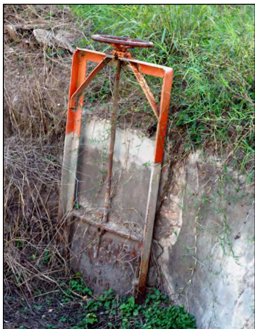
Figure 4.68 An example of a concrete turnout with an iron slide gate. The drawing below shows an older version of the same style and use (Texas). 259
