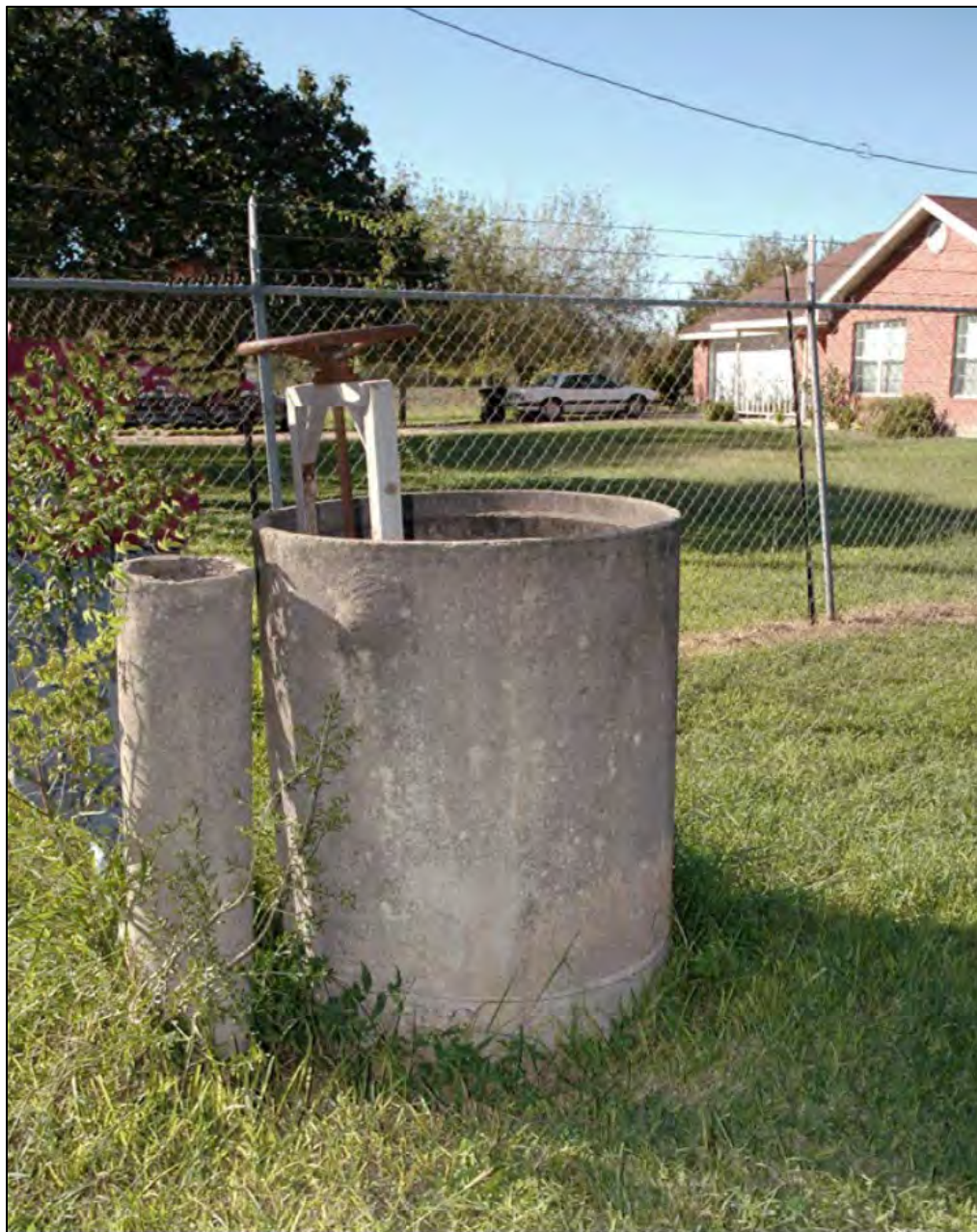
Figure 4.52 The vent is shown on the left. The large pipe protects the diversion stand valve in this Cameron County Irrigation District on Rio Grande Project (Texas). 245
