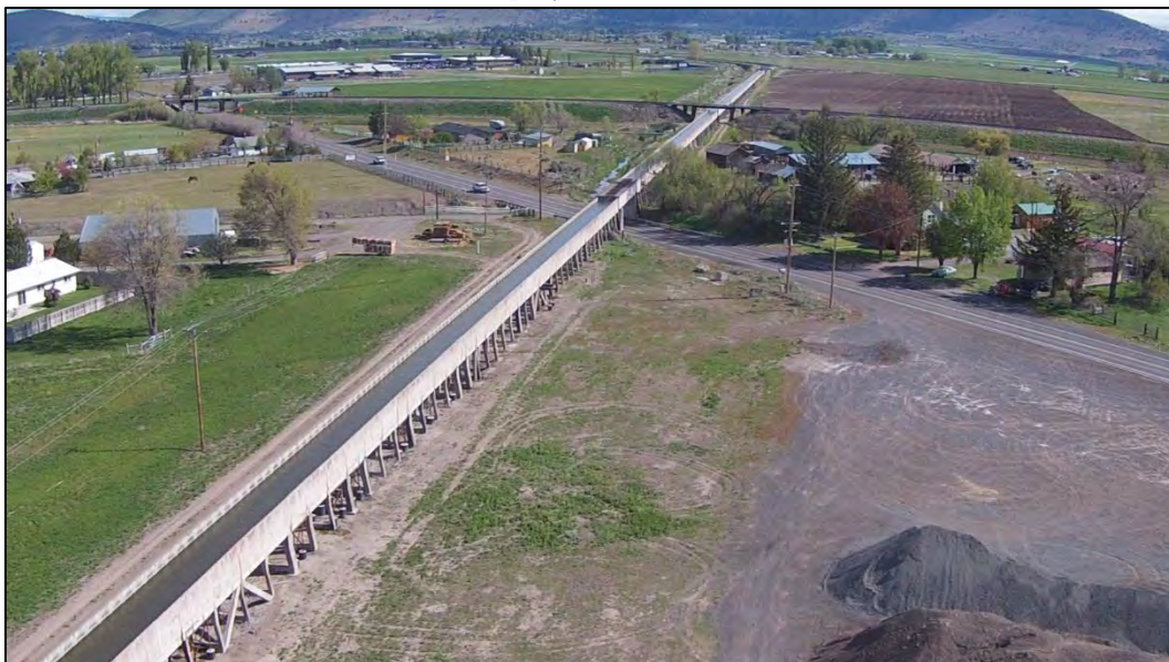
Figure 4.39 A concrete C Flume on a concrete pier foundation in the Klamath Project (Oregon and California). 233
