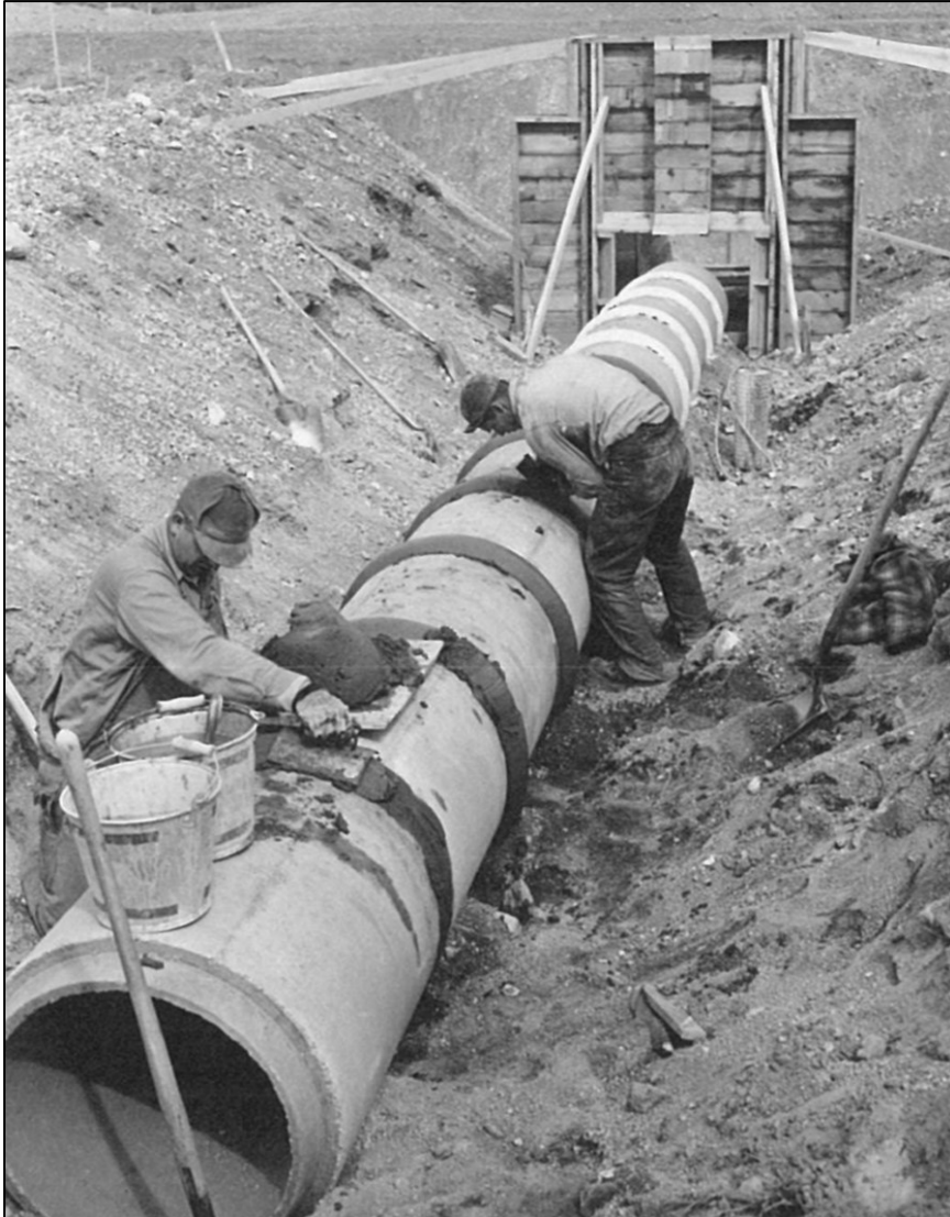
Figure 4.49 A photograph of the East Low Canal Section of concrete piping on the Columbia Basin Project (Washington State) in 1950. 242
