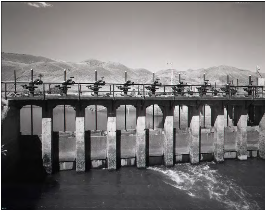
Figure 4.59 An excellent example of a concrete diversion dam with iron headgates on an unknown Reclamation project (courtesy of Bureau of Reclamation).
