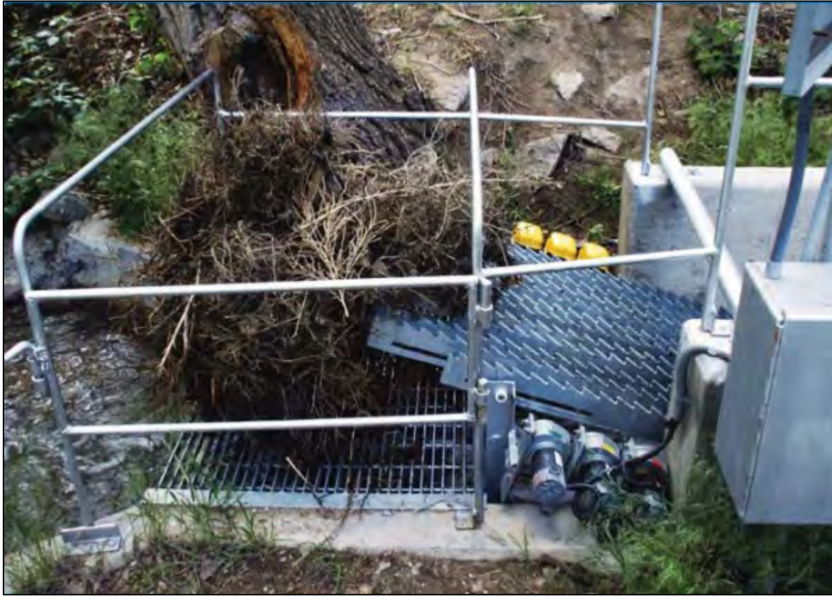
Figure 4.113 A self-cleaning metal trash rack being installed over an older drainage ditch trash gate on the Tetsel Ditch Project (Arizona; non-Reclamation Project). 313
