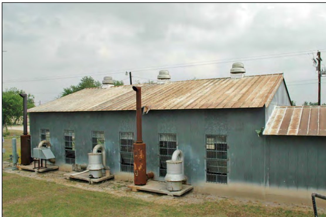
Figure 4.16 Metal pump station in the United Irrigation District, Lower Rio Grande Project (Texas). 214
