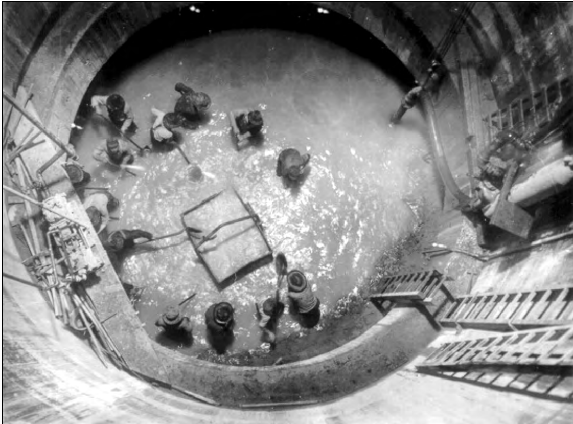
Figure 3.12 Yuma Project. Colorado River Siphon; looking down Arizona shaft 55 feet below surface at night, 1910 (courtesy of Bureau of Reclamation).
