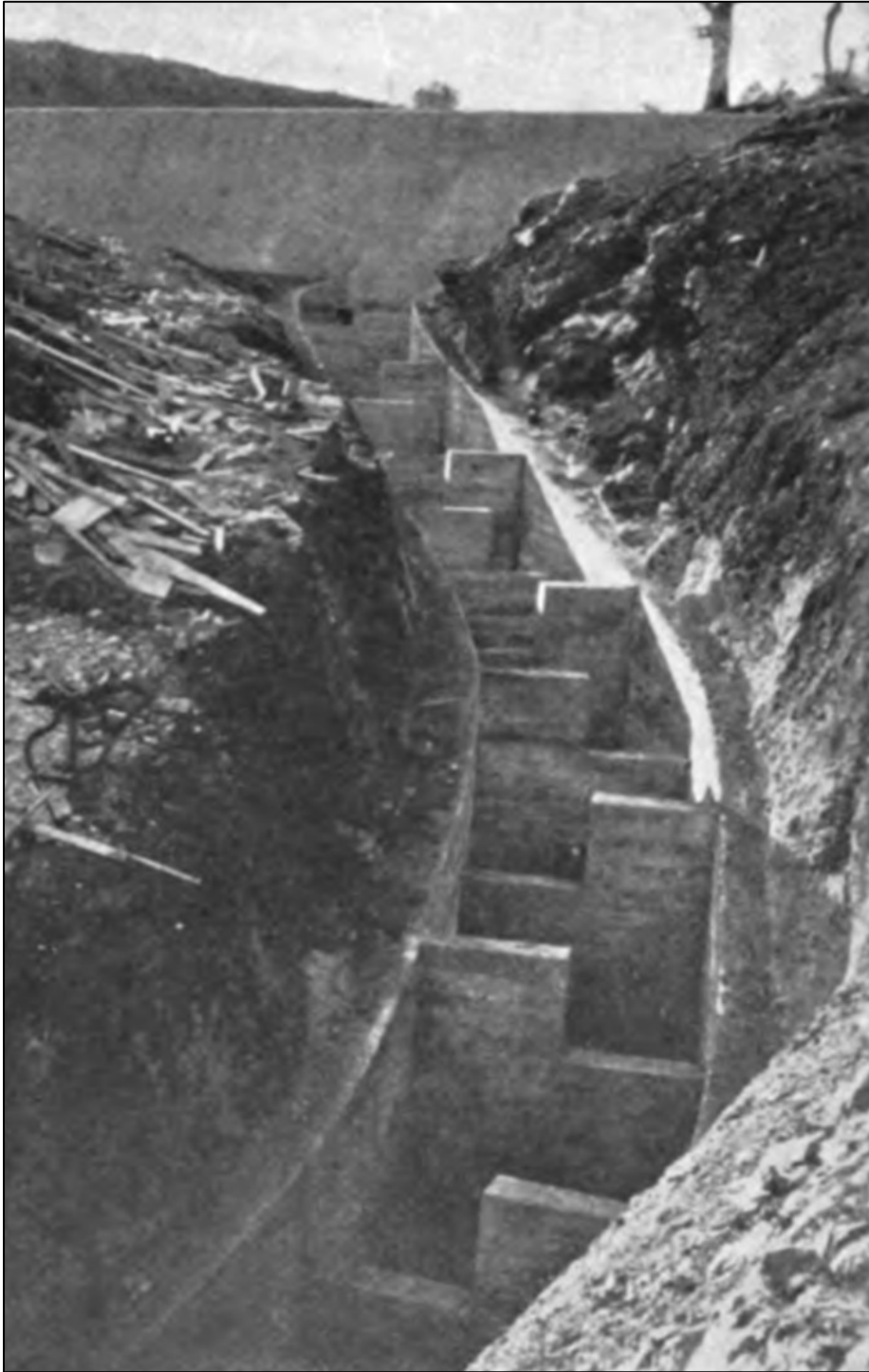
Figure 4.136 An early pool and traverse fish passage with baffles on the Feed Canal on the Orland Project. 336
