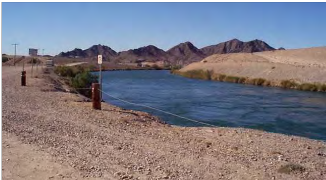
Figure 4.23 An unlined section of the All-American Canal (Arizona), partly lined and partly unlined in the Boulder Canyon Project, was completed in 1942 (courtesy of Bureau of Reclamation).
