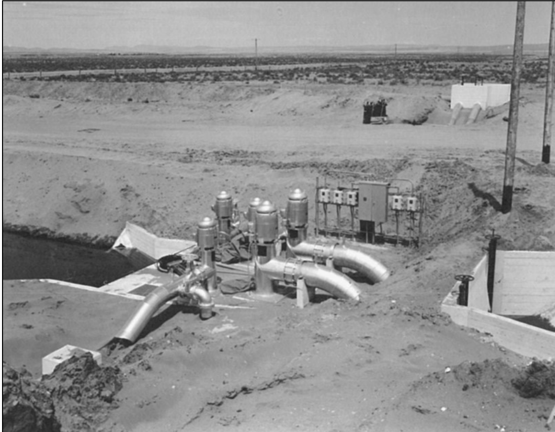
Figure 4.19 Uncovered pumping station on the Columbia Basin Project, Irrigation Division (Washington State), Burke Pump Plant, 1954. 218
