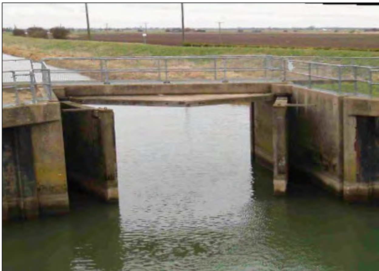
Figure 4.71 An example of a vertically hinged concrete headgate in a lateral on an unknown Reclamation Project. 262
