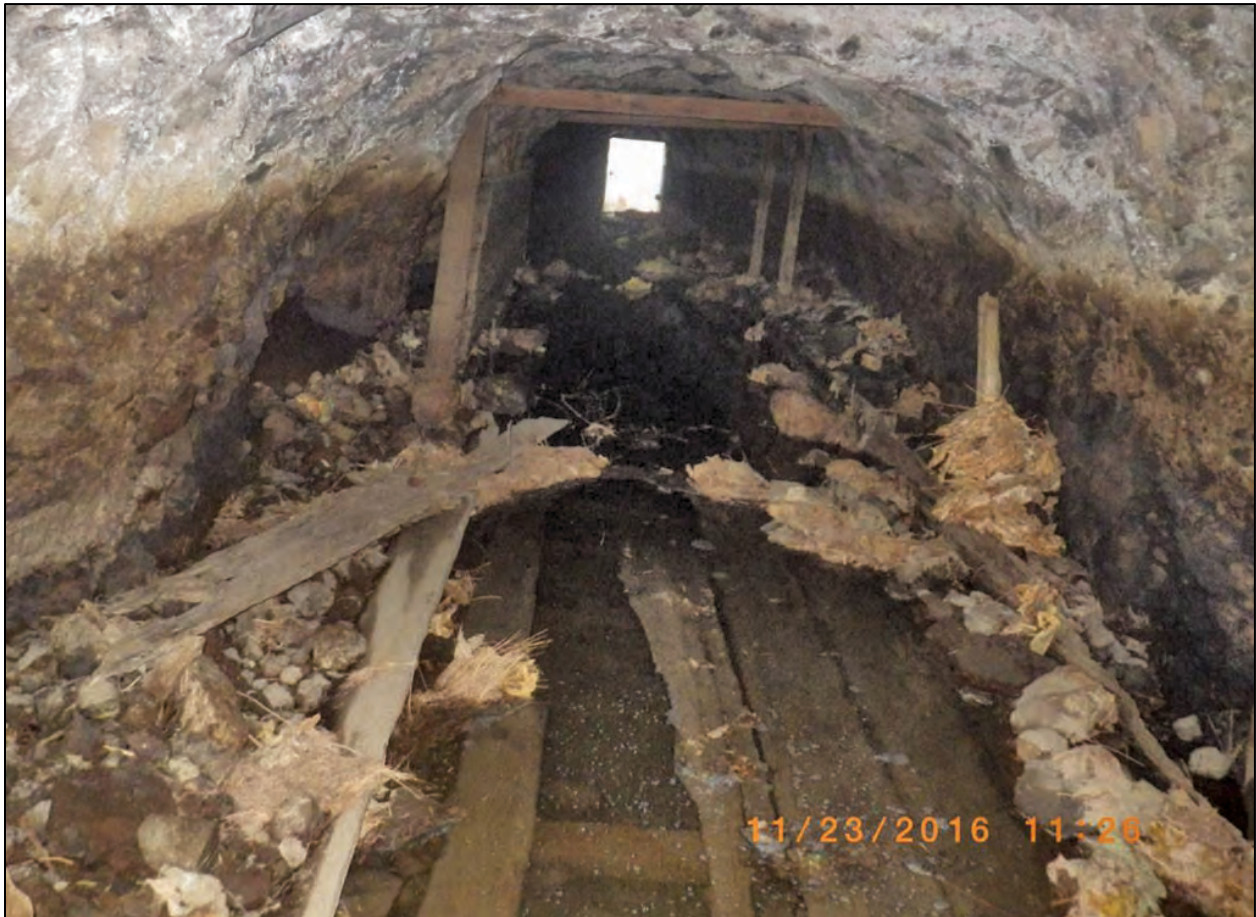
Figure 4.36 In need of repair, the wooden Pacific Tunnel inside the El Dorado Irrigation District in the CVP, California, is shown in 2016. 230
