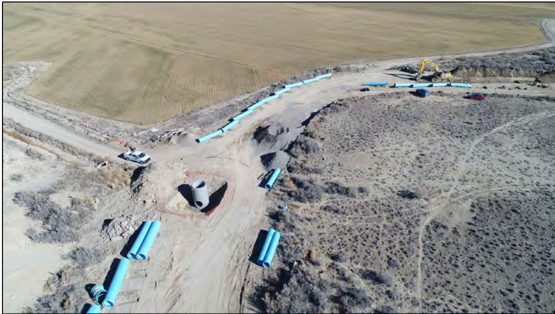
Figure 5.2 Recent piping of the GK Lateral of the Gunnison River Project (Colorado). 353
