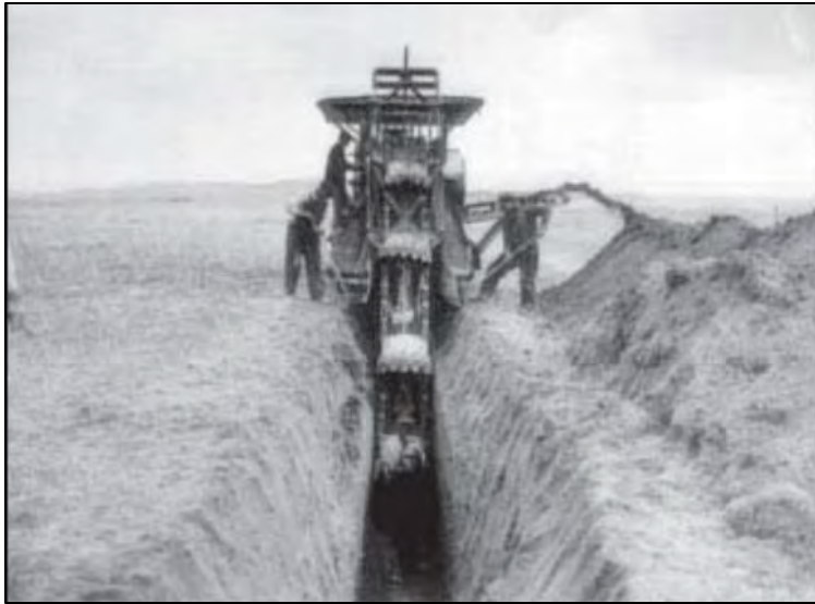
Figure 2.4 An auger digging a drainage ditch on the North Platte Project in Montana in 1917. Reclamation quickly discovered that drainage could be as serious a problem as not enough water. 36
