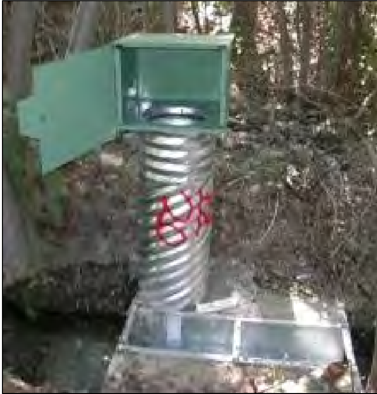
Figure 4.100 A metal stilling well placed into an irrigation system on an unknown Reclamation project (courtesy of Bureau of Reclamation).
