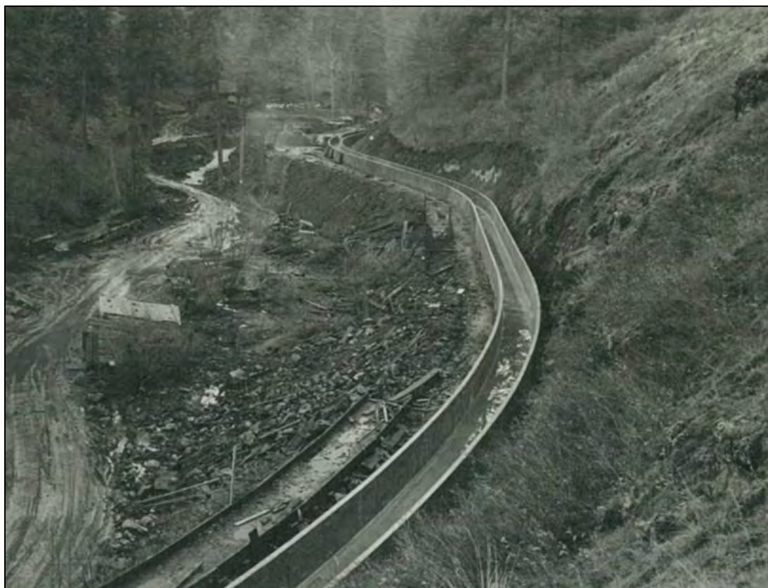
Figure 3.17 Lewiston Orchards Project main canal wooden flume being replaced with a concrete flume in 1948. 175
