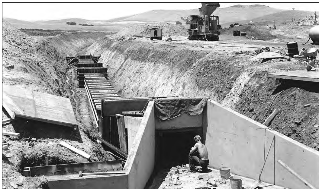
Figure 4.44 A large siphon being constructed to carry water underneath the Friant Kern Main Canal in the CVP (California). 238
