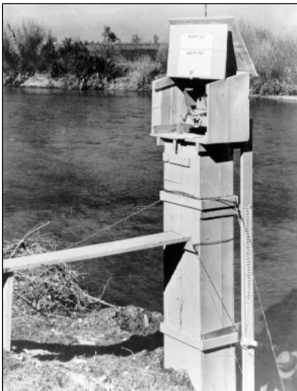
Figure 4.99 Wooden top of a stilling well showing the instrument for measuring water height in a Parshall flume on an unknown Reclamation project. 299
