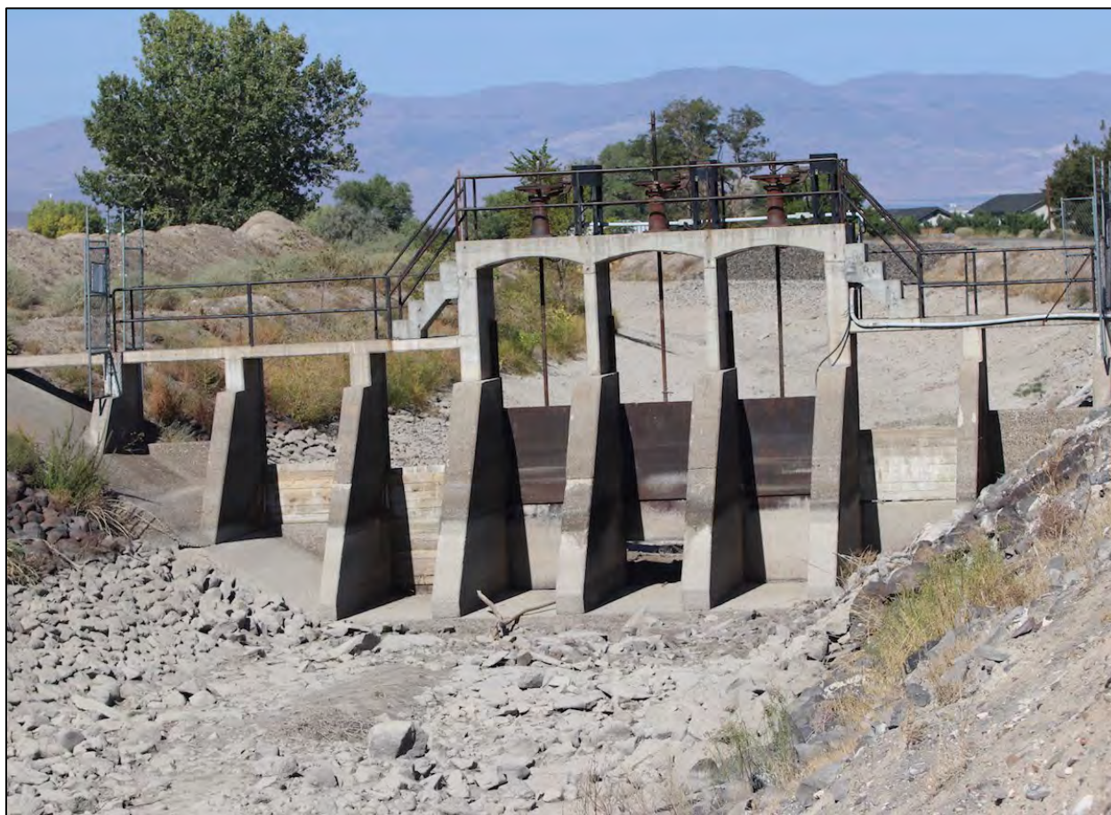
Figure 4.70 Concrete and cast-iron headgate on the Truckee Canal on the Newlands Project (Nevada). 261
