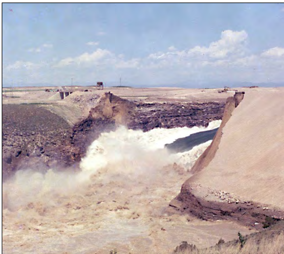
Figure 2.15 The catastrophic failure of the Teton Dam on June 5, 1976, on the Teton Valley Project. 90
