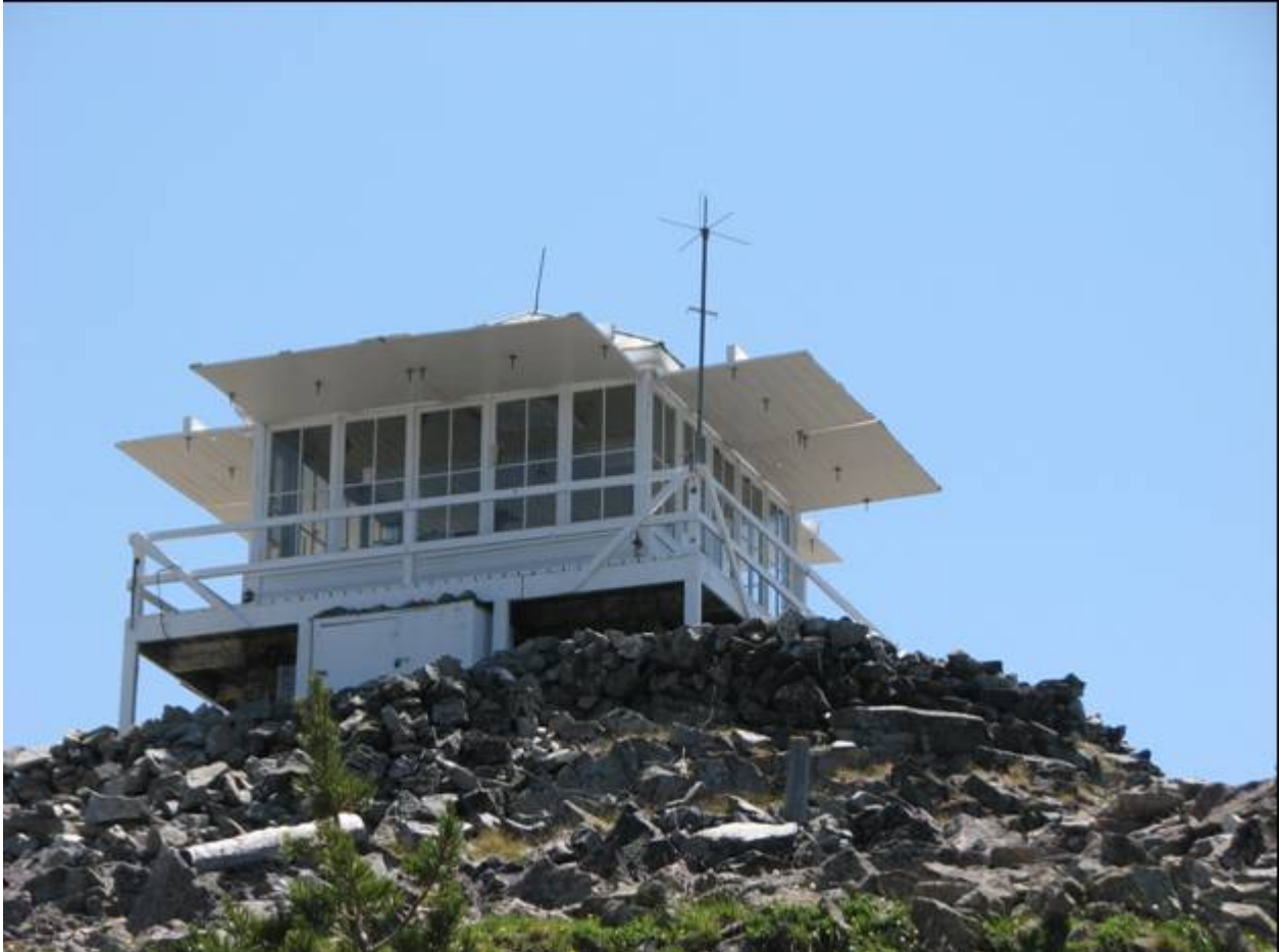
ID_IdahoCounty_Salmon Mountain Lookout_0002. Lookout and storage shed, looking south to the north and west walls of the lookout.
