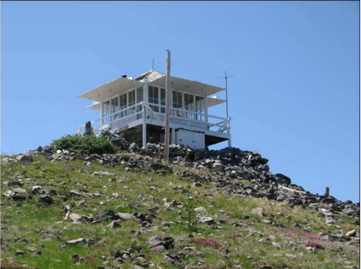
ID_IdahoCounty_Salmon Mountain Lookout_0001. Lookout and storage shed, looking southwest to the east (front) and north walls of the lookout.
