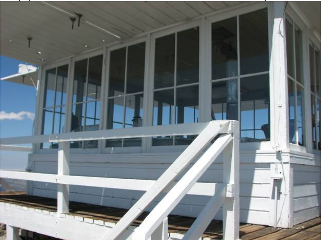
ID_IdahoCounty_Salmon Mountain Lookout_0003. Lookout, looking east-northeast to the south wall of the lookout.
