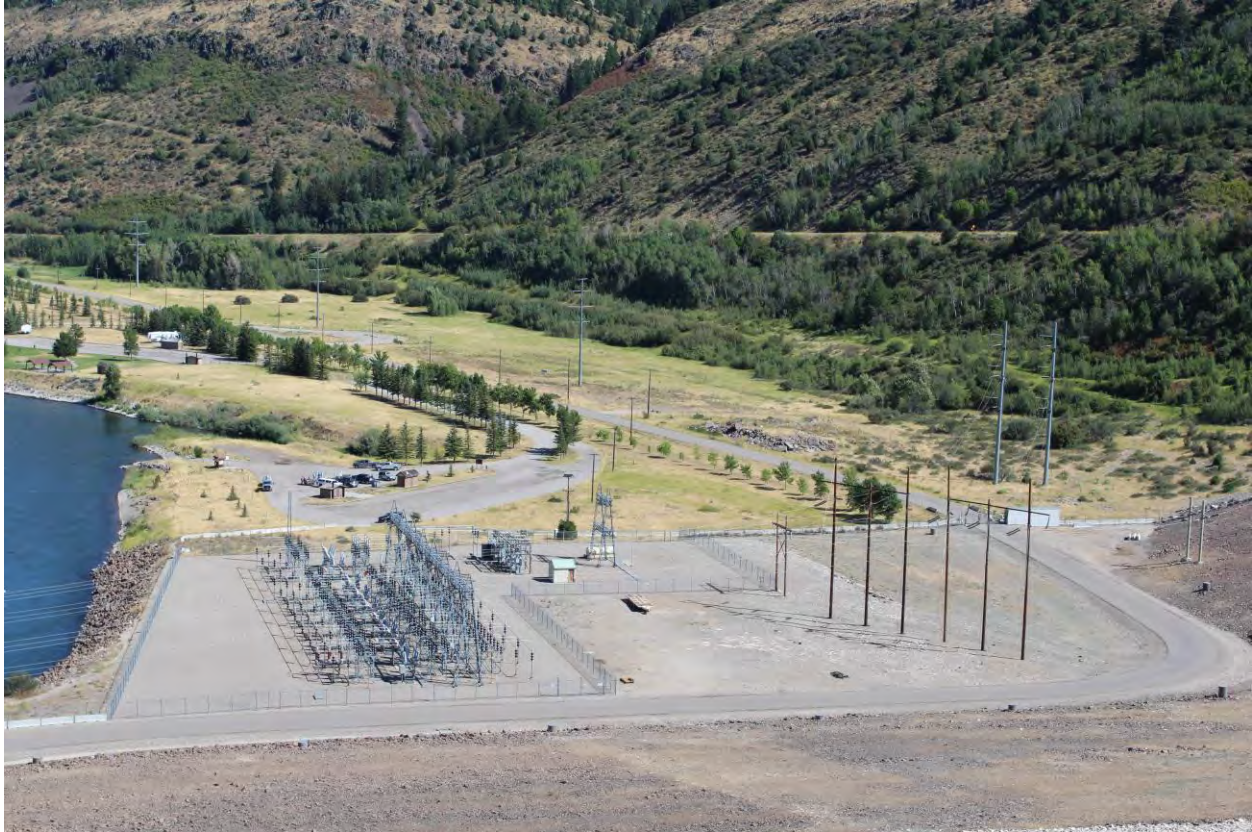
Photo 28 of 30. Switchyard and Access Road. View to north.
