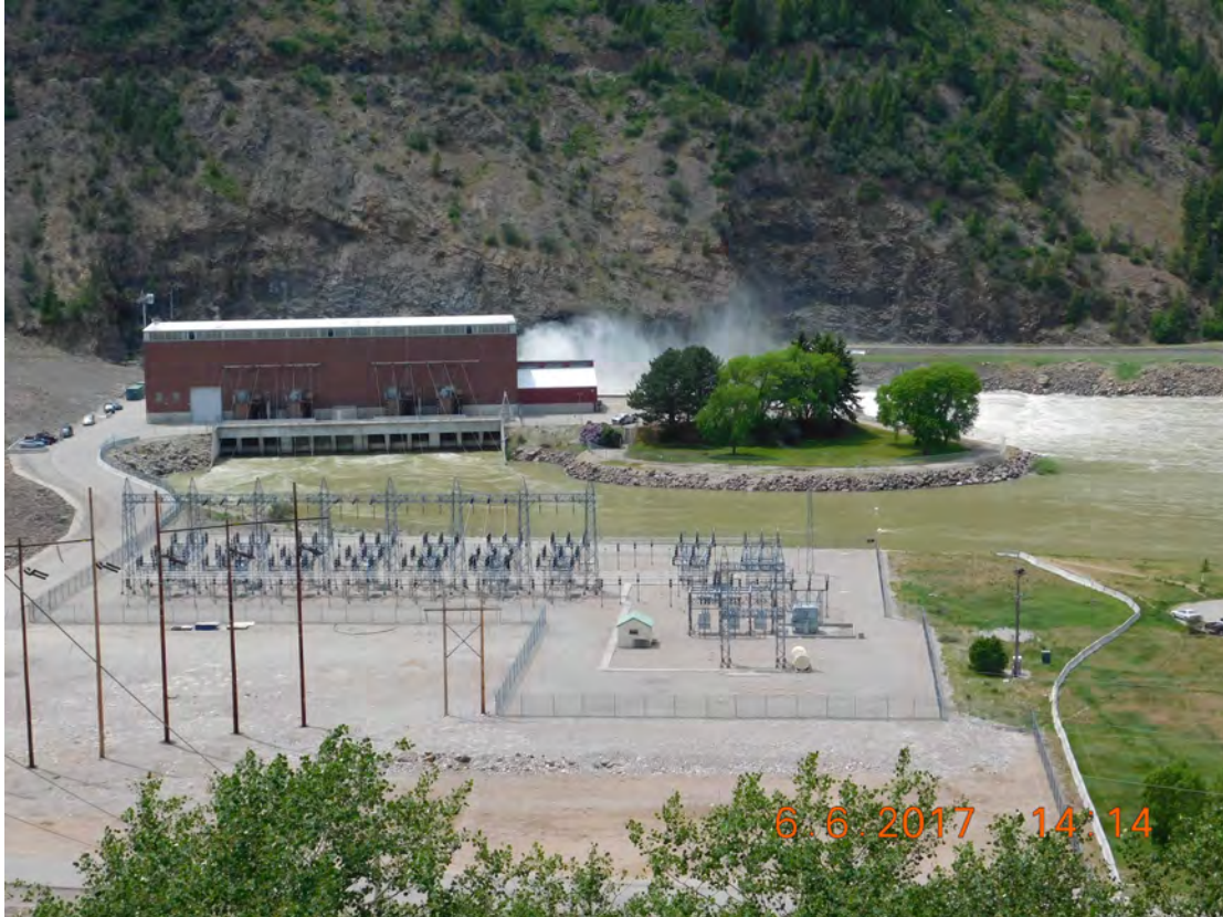
Photo 30 of 30. Vista Park on Right, Switchyard in Foreground Powerhouse to the Left. View West.
