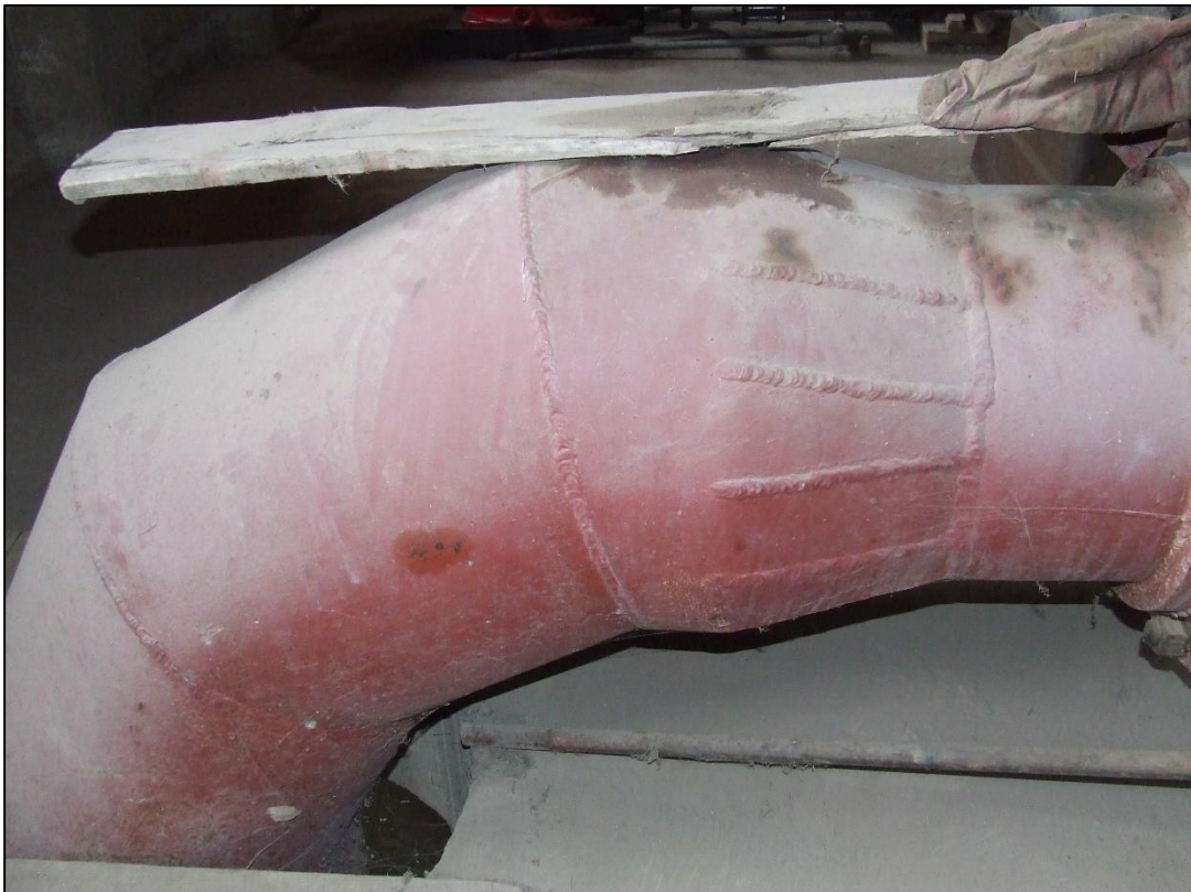
Photograph 16 of 25 Close up of inlet pipe for pump
