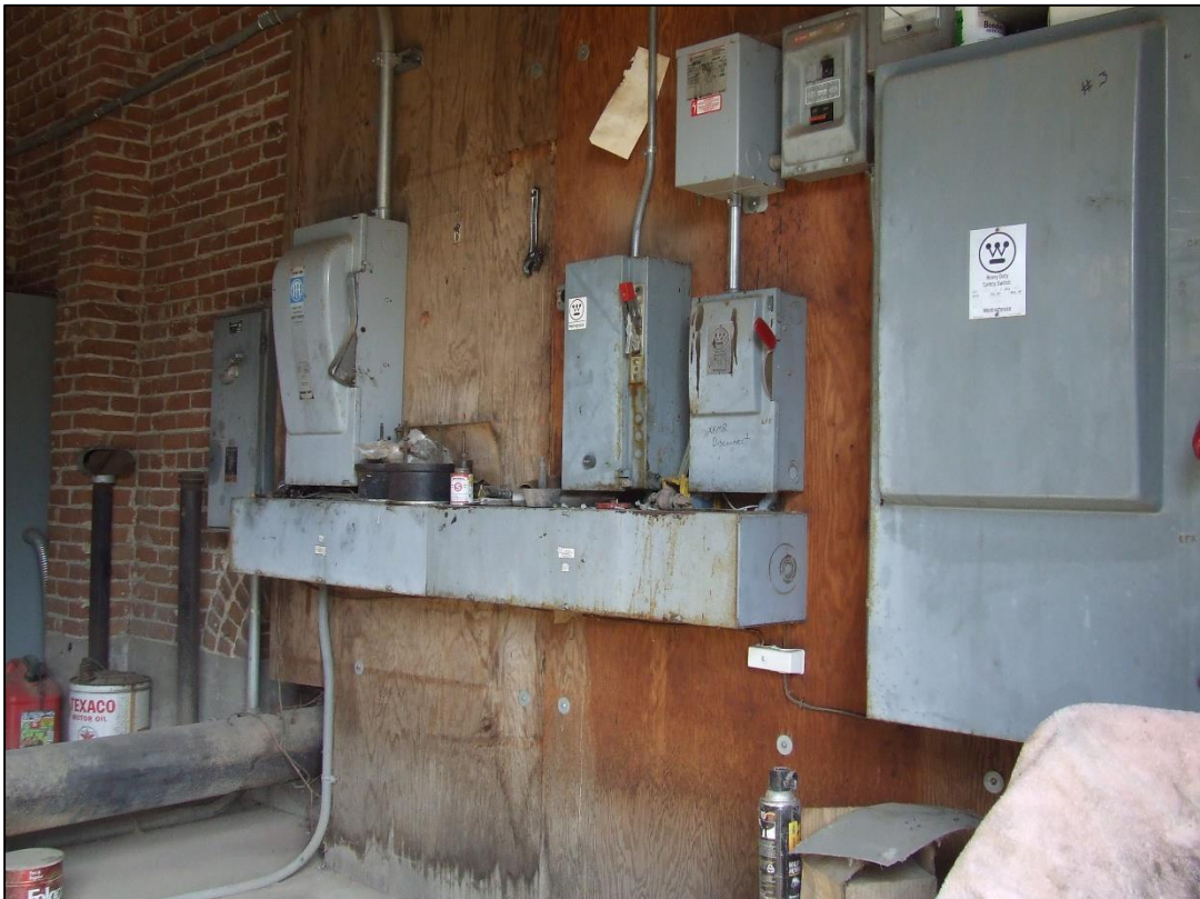
Photograph 22 of 25 Switch boxes mounted on north wall
