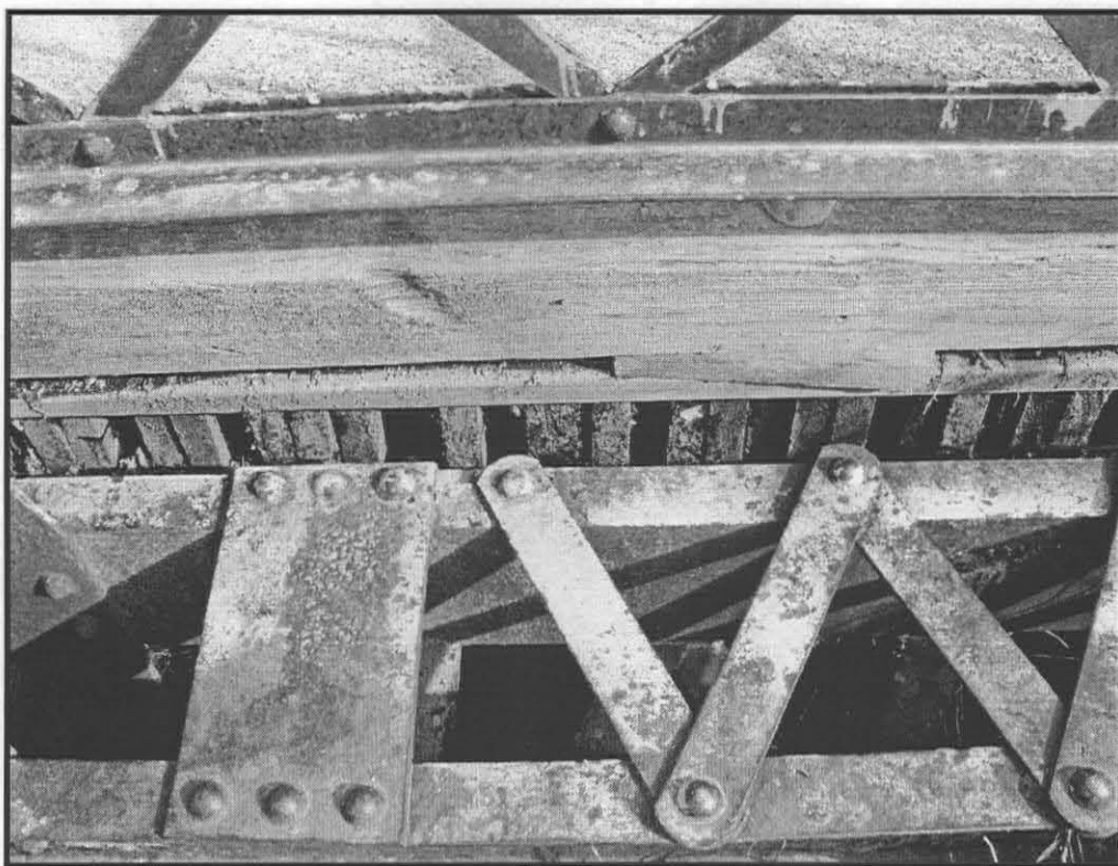
Webbed truss detail adjacent to wood deck and bottom of guard rail.
