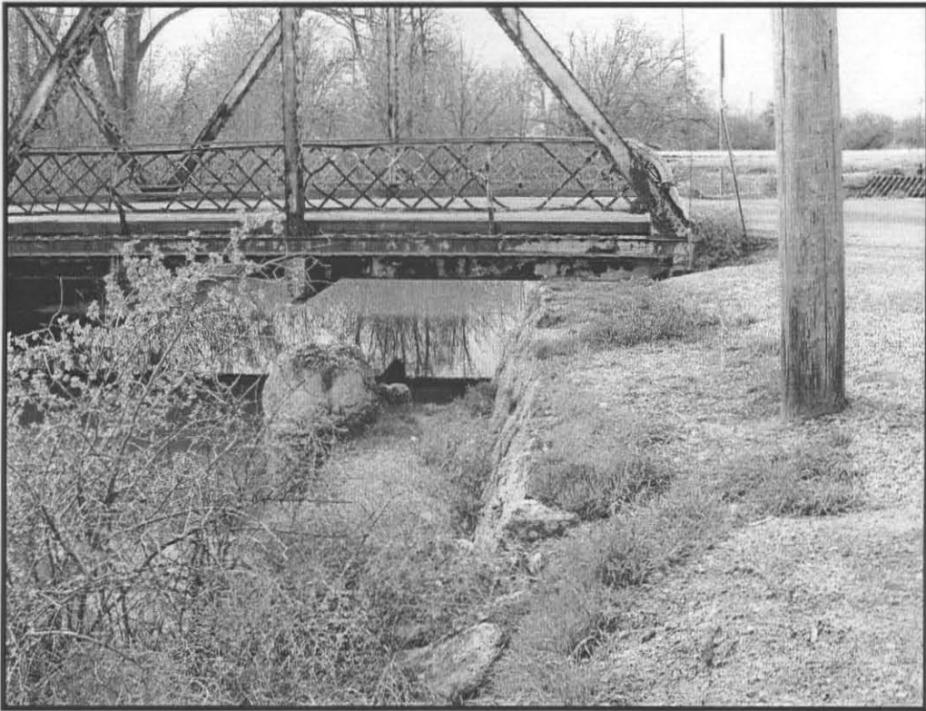
Boise River and Canal Bridge east side abutment and former bridge masonry abutment. Viewed to the south.
